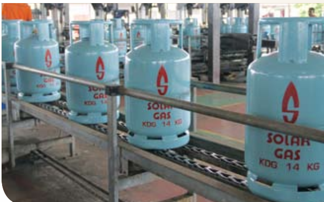
OIL & GAS/ENERGY SECTOR: Summit Petroleum LPG Cylinder Filling Plant at West Port, Klang
