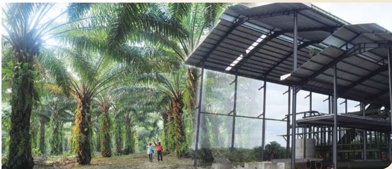
AGRO BUSINESS SECTION: KUB Agro Holdings' oil palm estate and mill (under construction)
