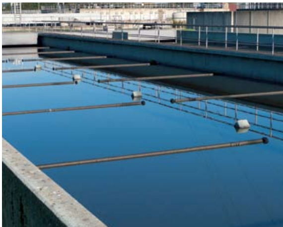
Binh An Water Treatment Plant, Vietnam
