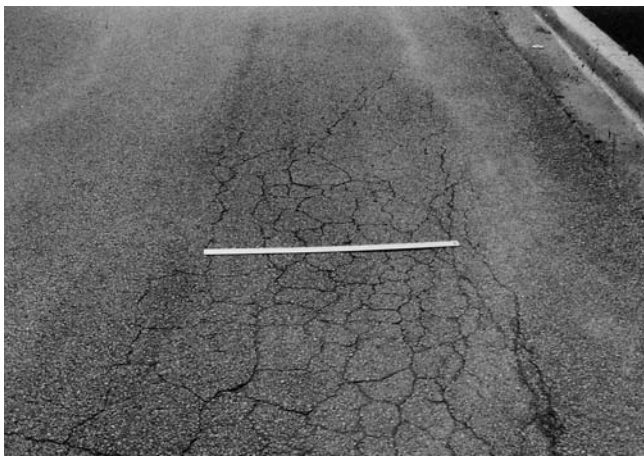
FIG. X1.2 Medium-Severity Alligator Cracking
