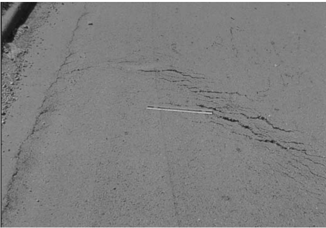
FIG. X1.48 Medium-Severity Slippage Cracking
