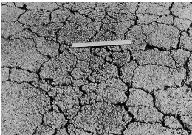
FIG. X1.3 High-Severity Alligator Cracking
