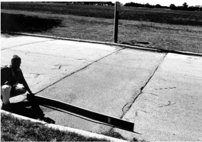
FIG. X1.32 Medium-Severity Patching and Utility Cut Patching
