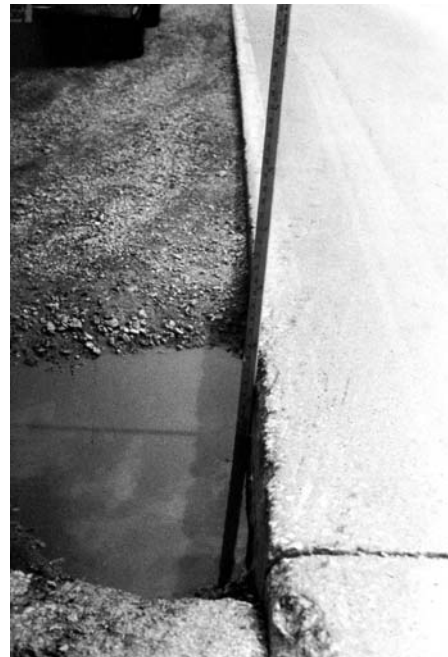
FIG. X2.21 High-Severity Lane/Shoulder Drop-Off
