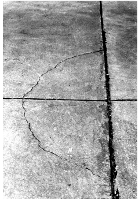
FIG. X2.4 Low-Severity Corner Break
