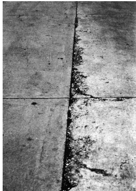
FIG. X2.49 Medium-Severity Spalling, Joint
