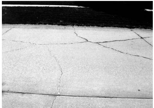
FIG. X2.8 Medium-Severity Divided Slab
