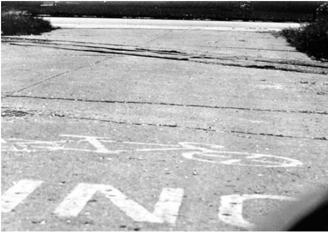
FIG. X2.39 Medium-Severity Railroad Crossing
