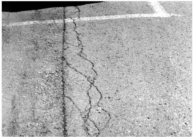
FIG. X1.20 Medium-Severity Edge Cracking
