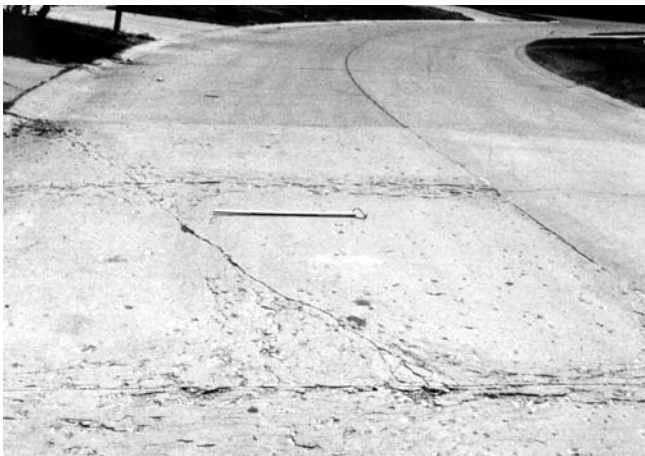
FIG. X2.12 High-Severity Durability Cracking
