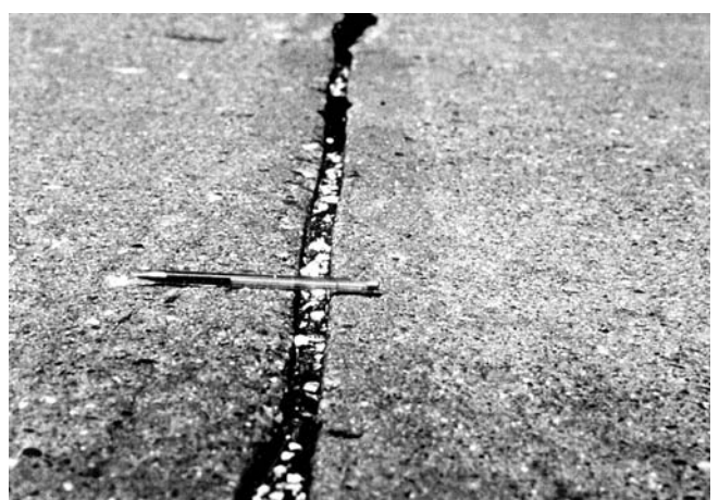
FIG. X2.18 High-Severity Joint Seal Damage
