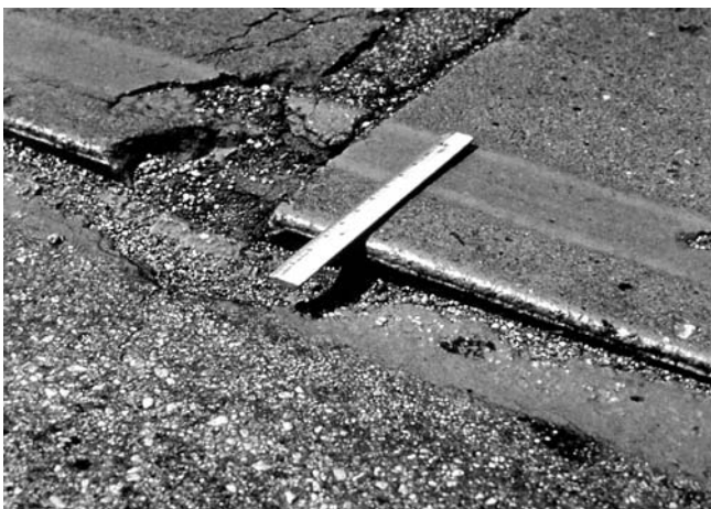
FIG. X2.19 Low-Severity Lane/Shoulder Drop-Off
