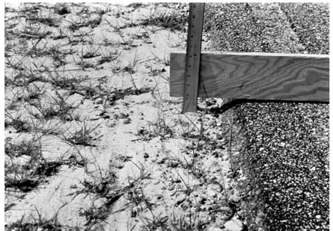
FIG. X1.25 Low-Severity Lane/Shoulder Drop-Off
