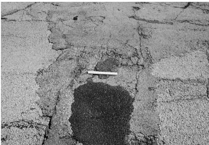
FIG. X1.33 High-Severity Patching and Utility Cut Patching
