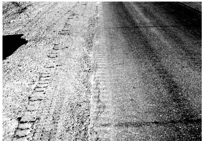
FIG. X1.22 Low-Severity Joint Reflection Cracking
