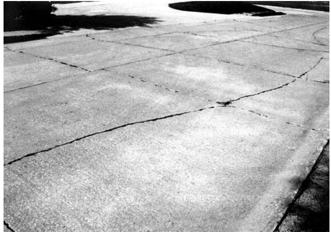
FIG. X2.7 Low-Severity Divided Slab
