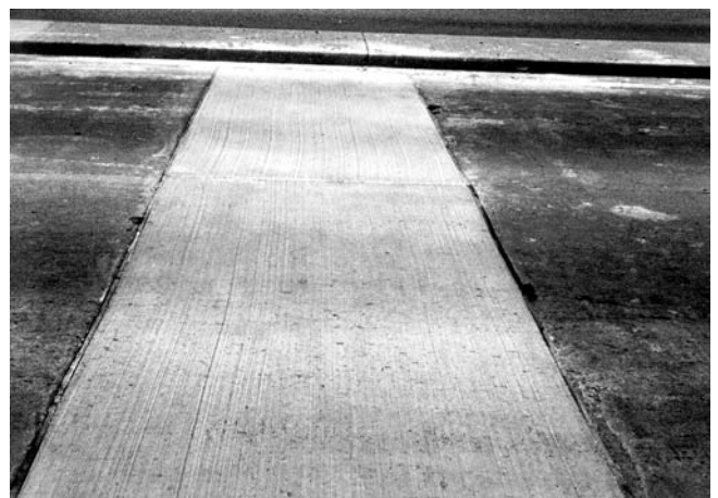
FIG. X2.25 Low-Severity Patching, Large and Utility Cuts
