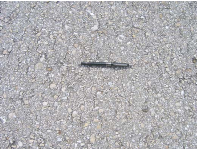
FIG. X1.53 Low-Severity Weathering (Surface Wear)
