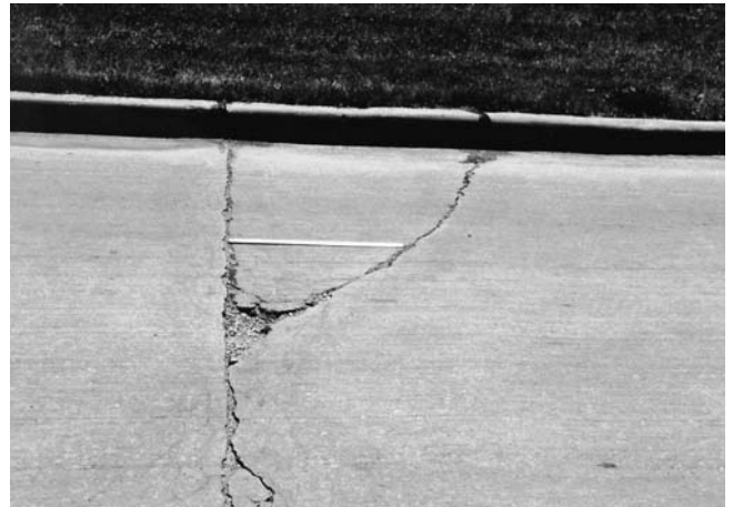
FIG. X2.5 Medium-Severity Corner Break
