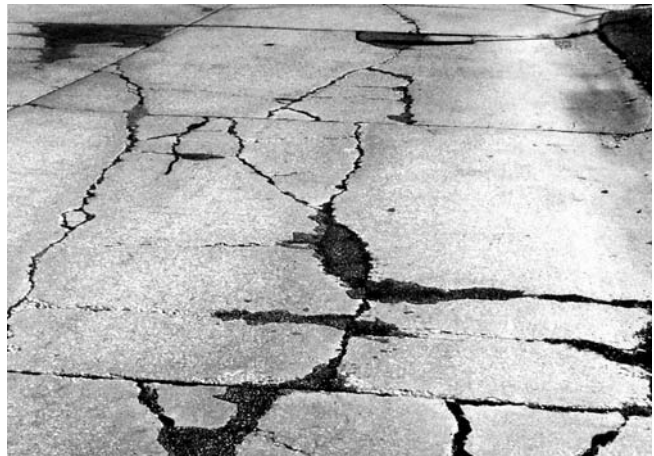
FIG. X2.9 High-Severity Divided Slab
