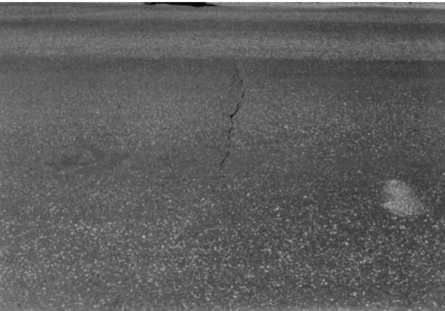
FIG. X1.28 Low-Severity Longitudinal and Transverse Cracking
