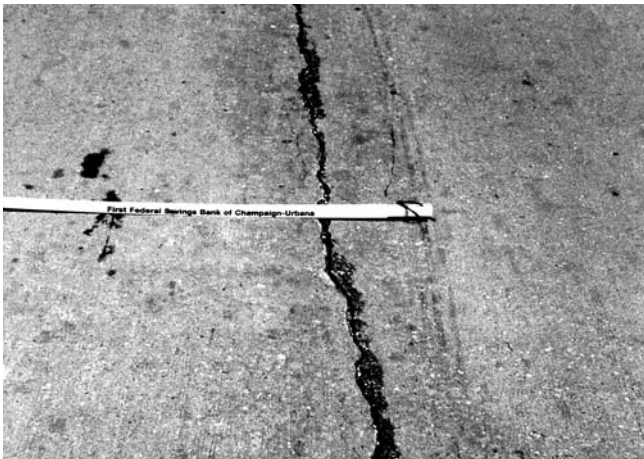
FIG. X2.23 Medium-Severity Linear Cracking
