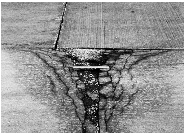
FIG. X2.11 Medium-Severity Durability Cracking
