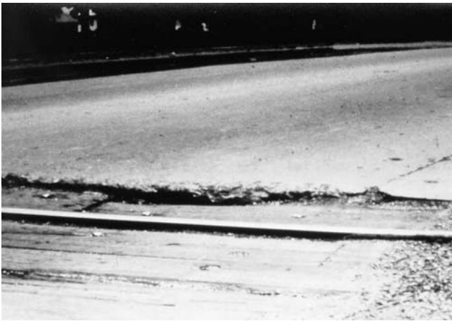
FIG. X2.40 High-Severity Railroad Crossing
