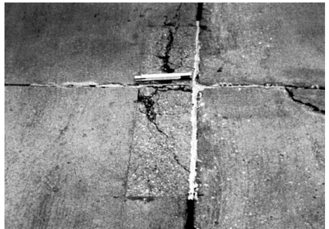
FIG. X2.30 High-Severity Patching, Small
