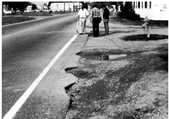
FIG. X1.21 High-Severity Edge Cracking
