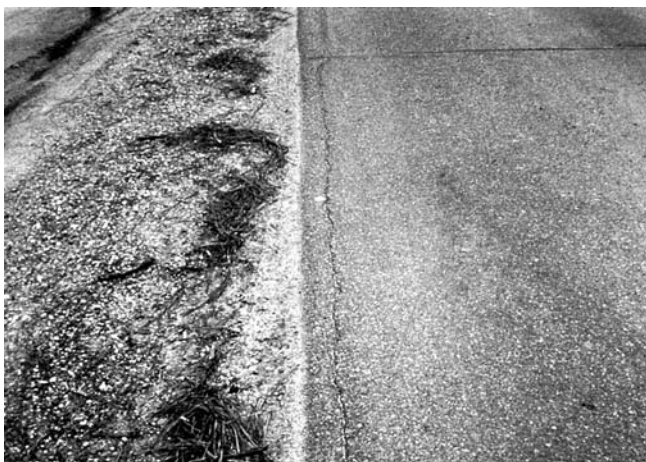
FIG. X1.19 Low-Severity Edge Cracking
