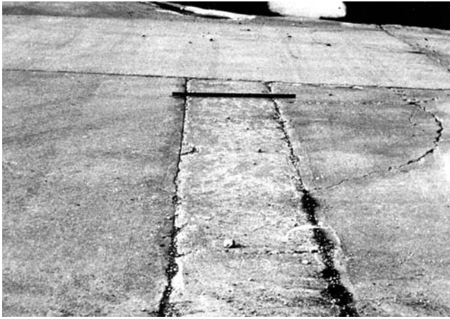
FIG. X2.26 Medium-Severity Patching, Large and Utility Cuts
