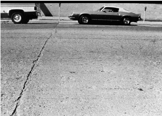
FIG. X2.48 Low-Severity Spalling, Joint
