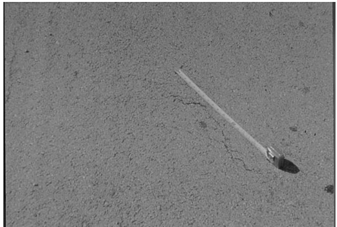
FIG. X1.47 Low-Severity Slippage Cracking
