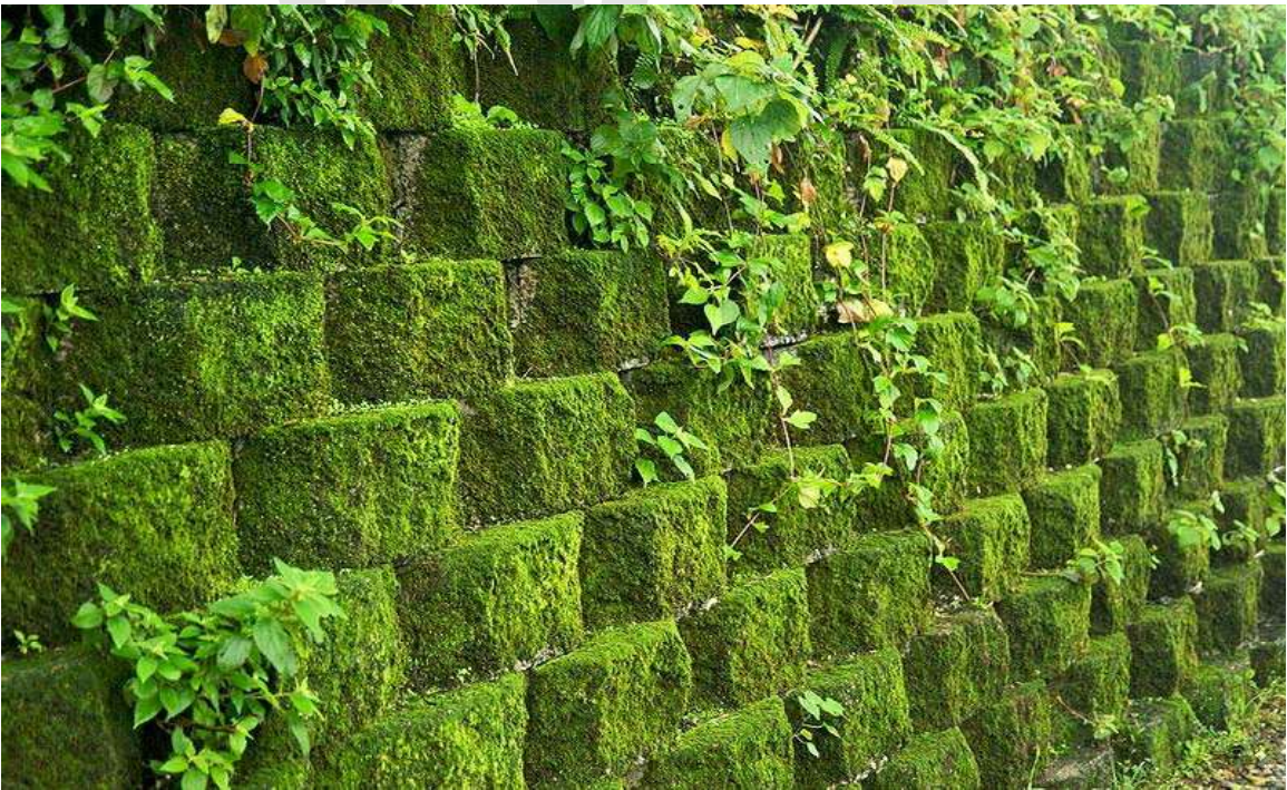
Retaining wall covered in moss
