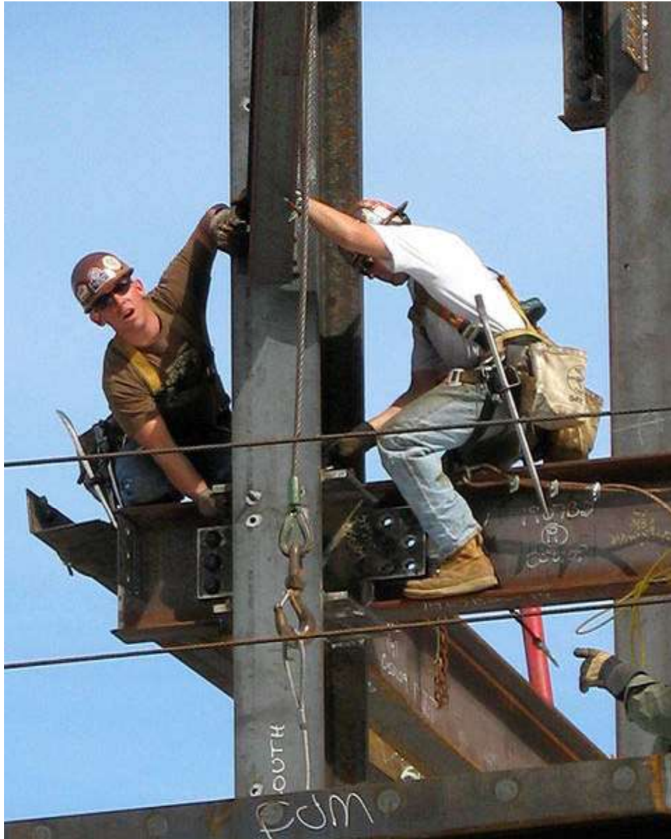
Ironworkers erecting the steel frame of a new building at Massachusetts General Hospital, Boston
