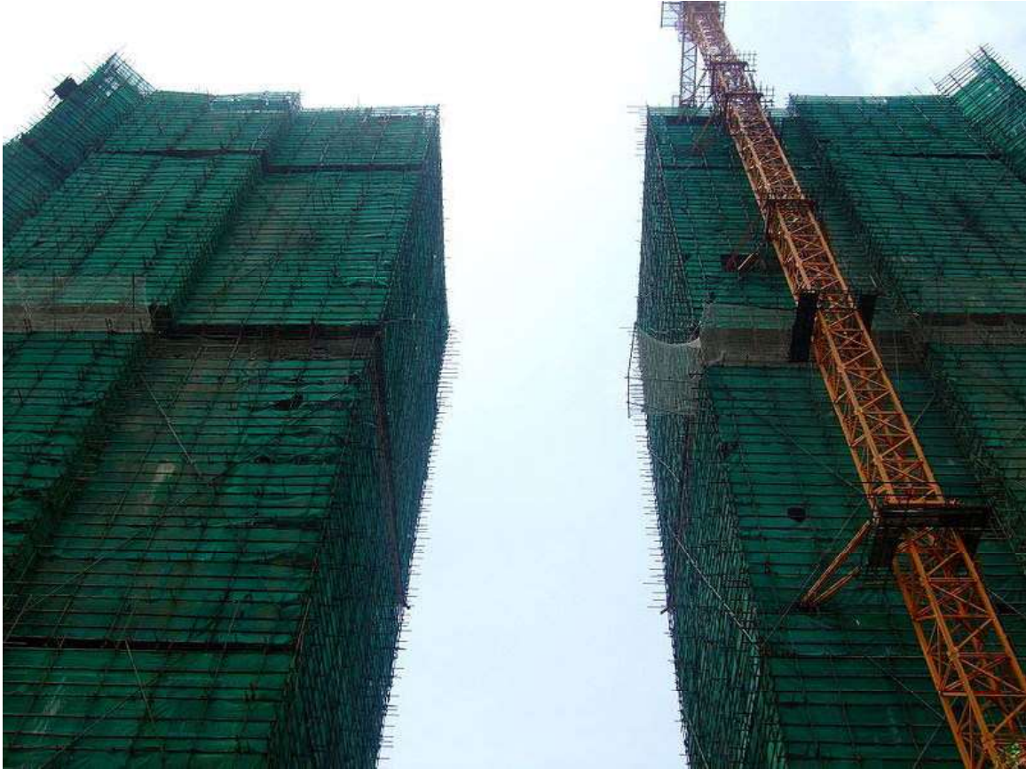
Construction of the Phase-1 (first two towers) of the Havelock City Project, Sri Lanka.
