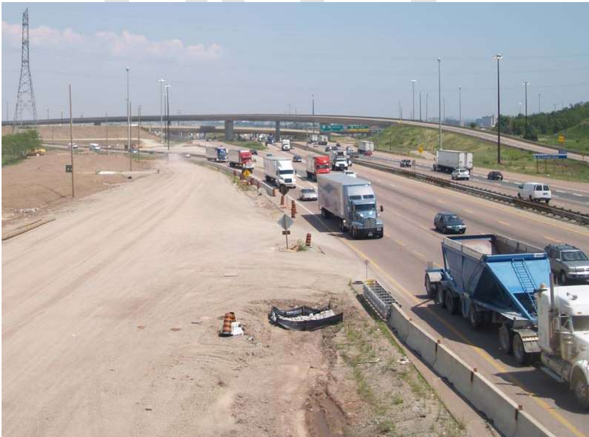
Construction along Ontario Highway 401, widening the road from six to twelve travel lanes.
