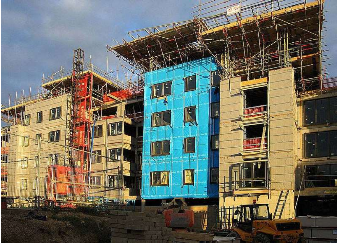
A building site for a row of riverside apartment blocks in Cambridge
