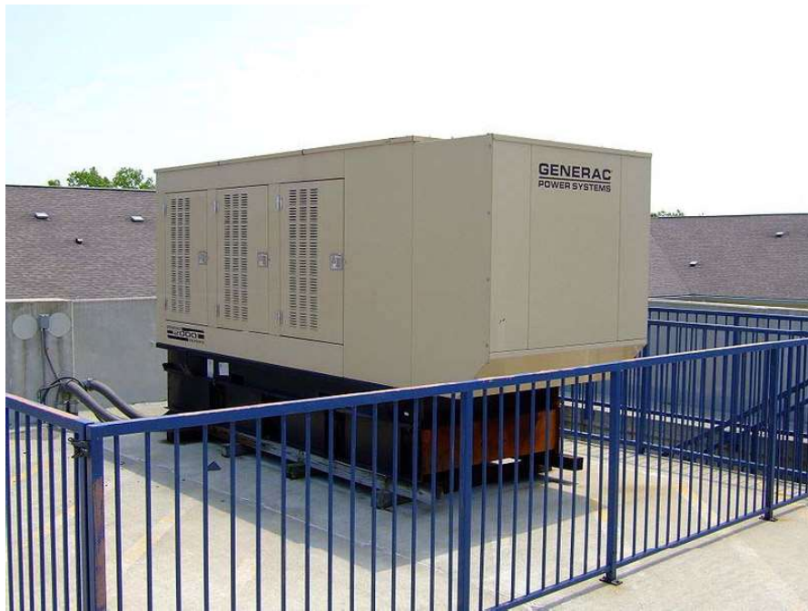
A backup generator for a large apartment building
