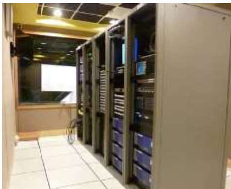
Central Apparatus Room (CAR)
