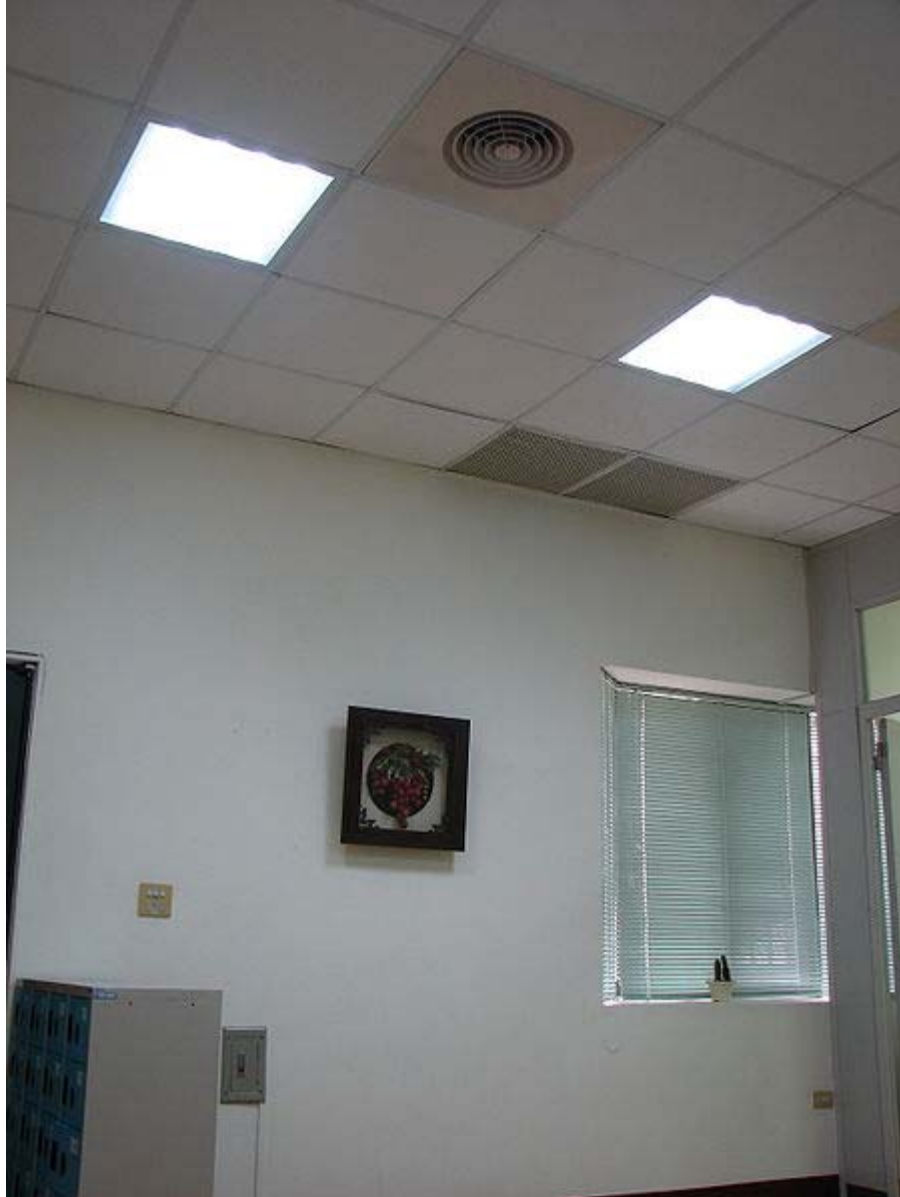
Dropped ceiling with LED lamps
