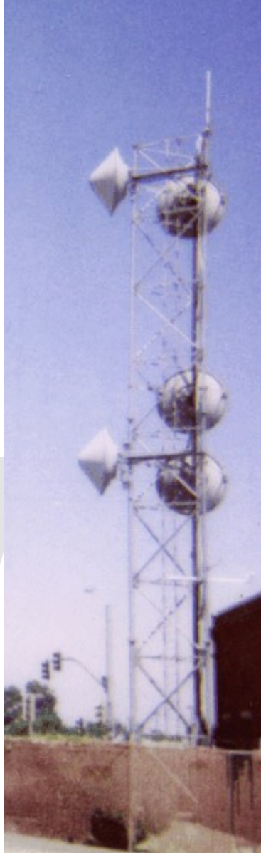
A terrestrial microwave radio antenna array
