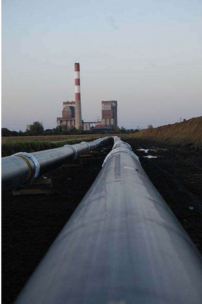
District heating pipeline in Austria with a length of 31 km
