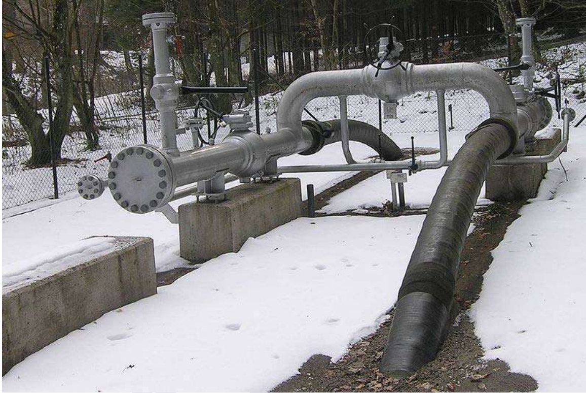
A "Pig" launcher/receiver, belonging to the natural gas pipeline in Switzerland.
