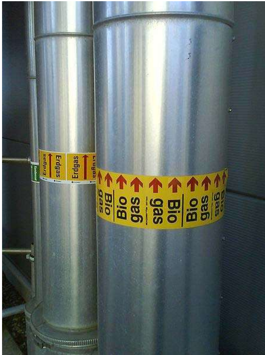
Biogas carrying pipes
