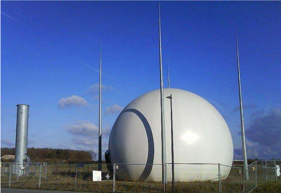
Biogas holder with lightning protection rods and back-up gas flare
