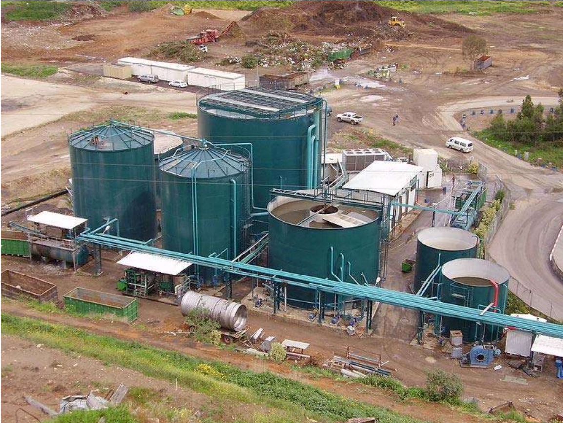
Two-stage, low-solids, UASB digestion component of a mechanical biological treatment system near Tel Aviv, process water is seen in balance tank and sequencing batch reactor, 2005
