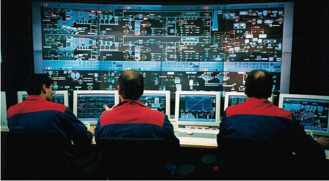
Control room of a typical moving grate incinerator overseeing two boiler lines
