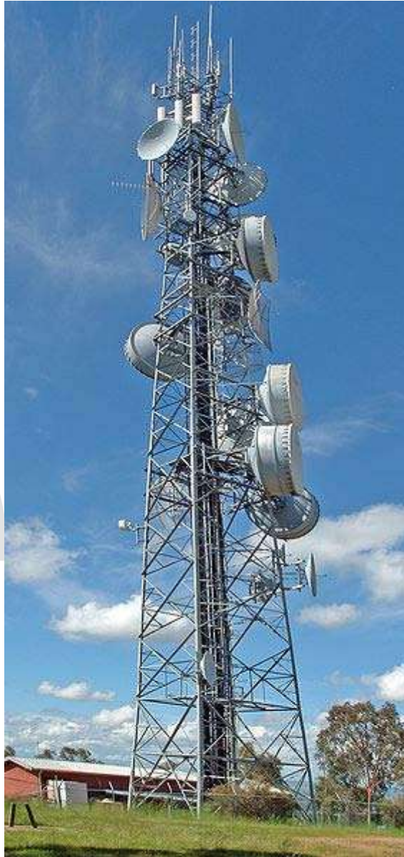
Steel lattice tower
