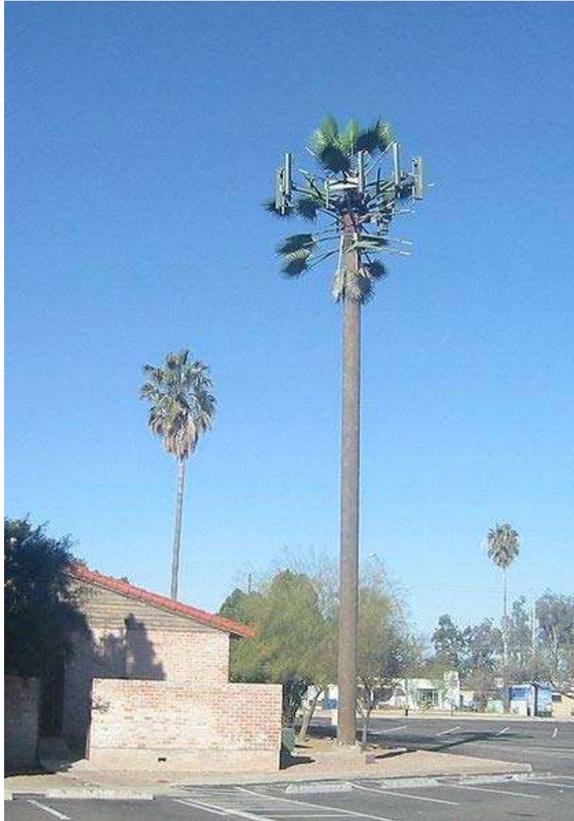
Telephone site concealed as a palm tree.
