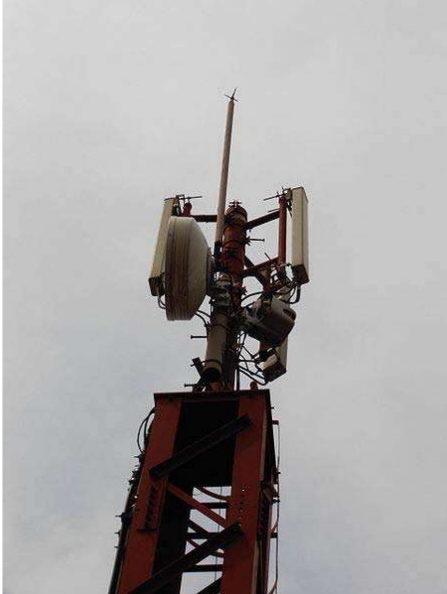
A three-sector telephone site in Mexico City.
