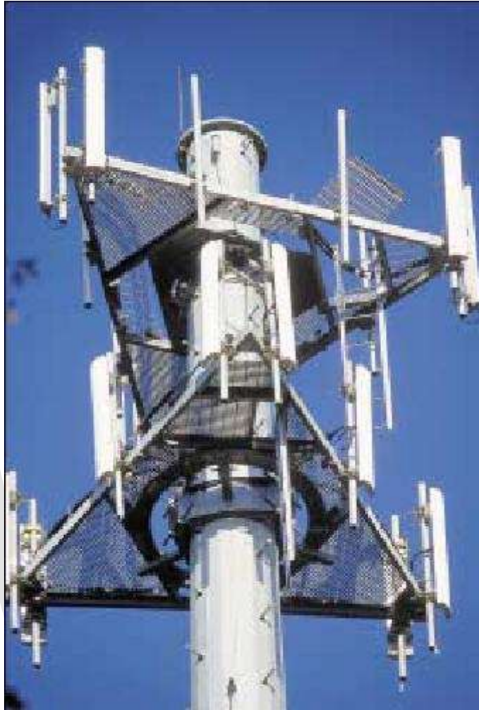
Cell phone base station antennas
