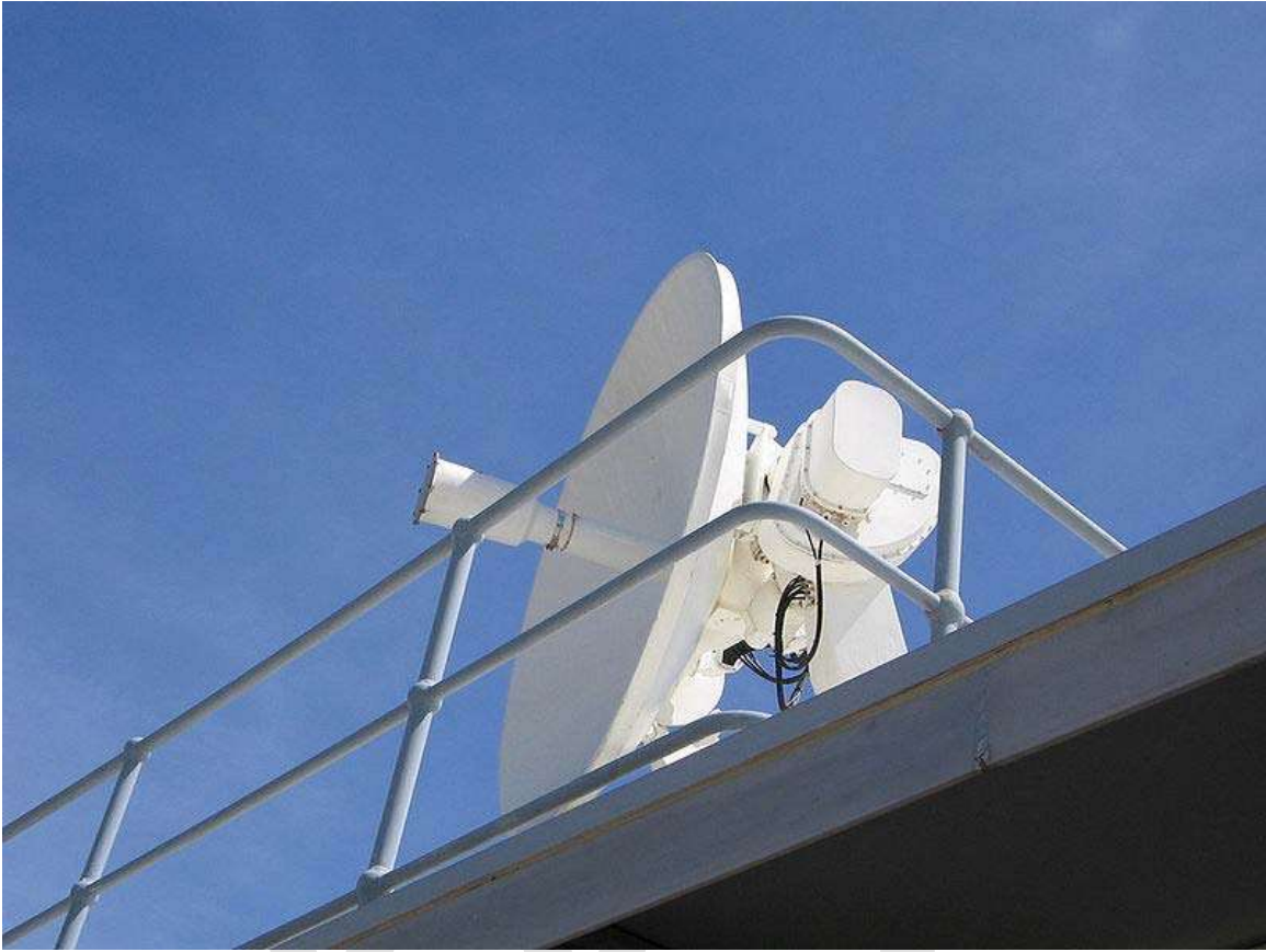
Weather (WF44) radar dish
