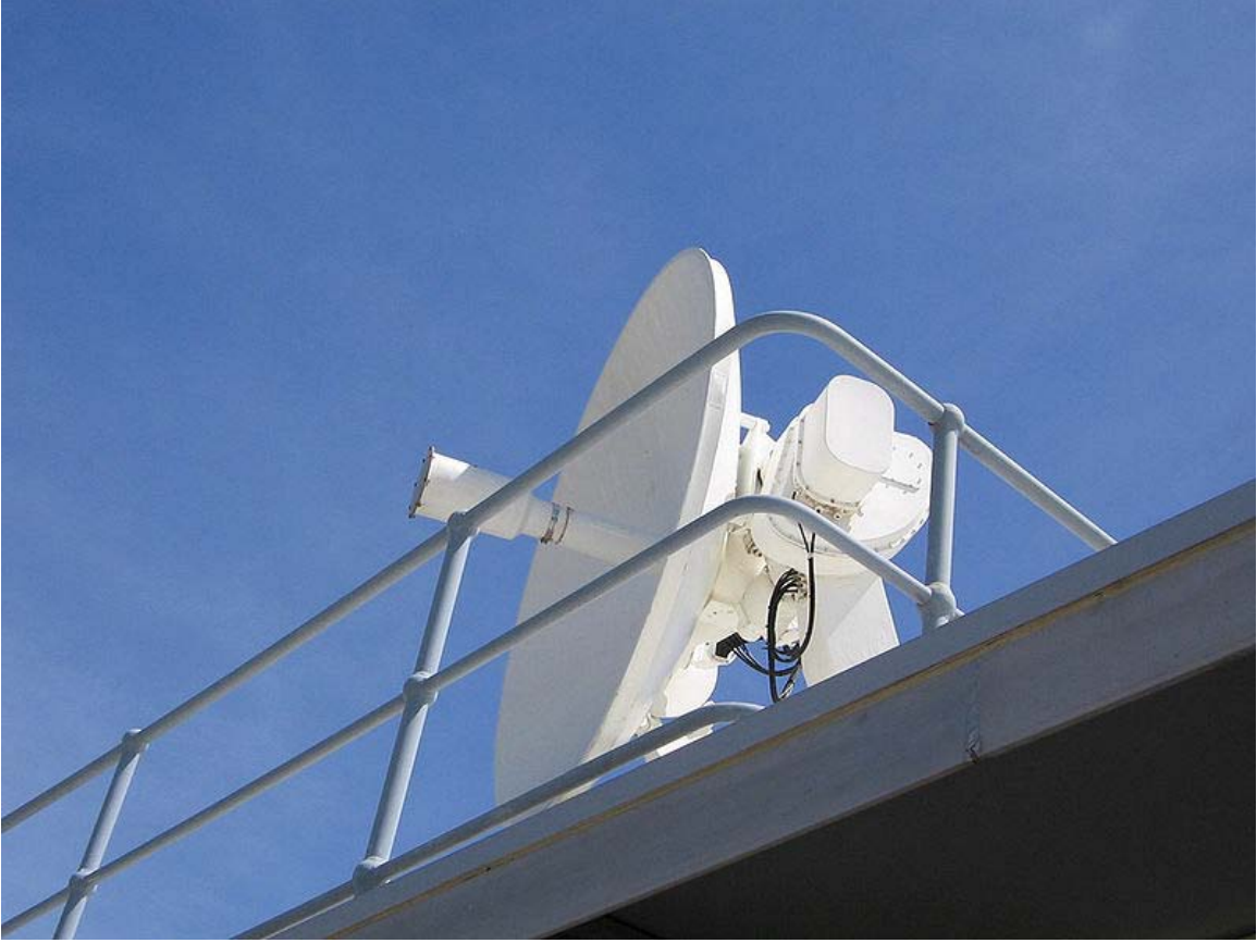
Weather (WF44) radar dish
