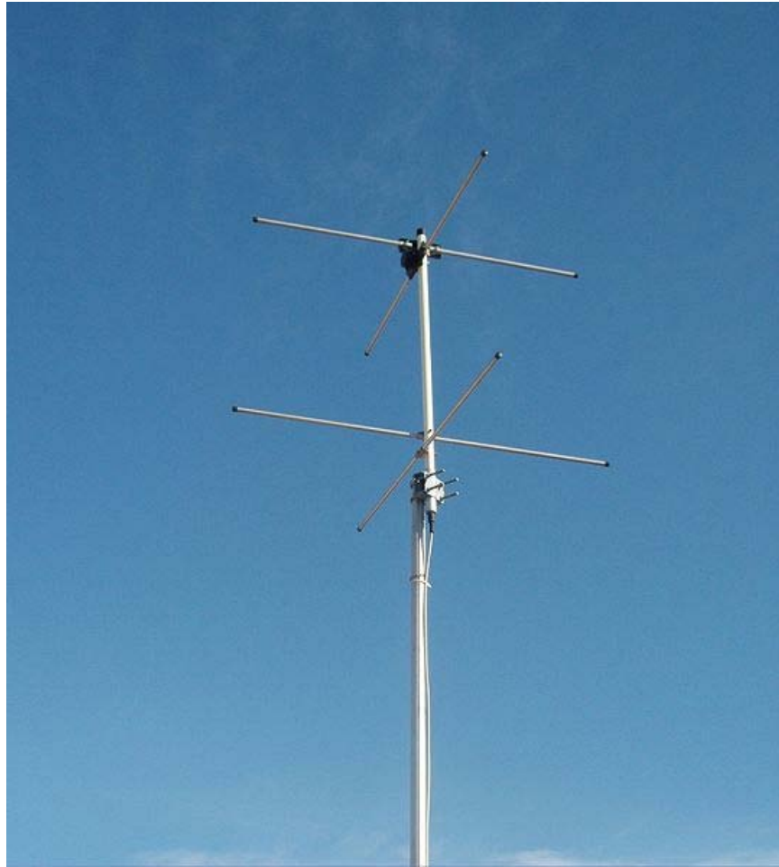
Turnstile antenna for reception of 137 MHz LEO weather satellite transmissions
