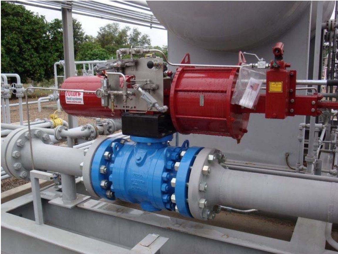
Pneumatically actuated shut down valve
