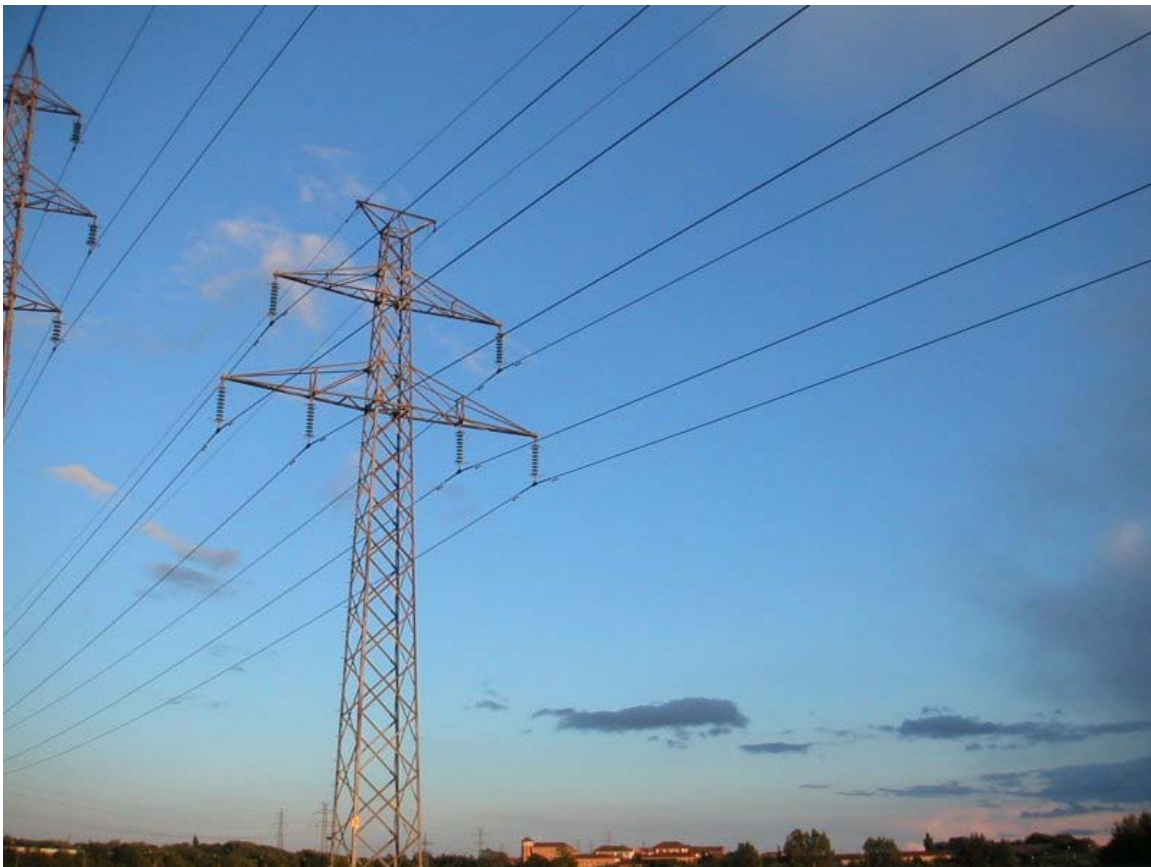
Transmission lines transmit power across the grid.
