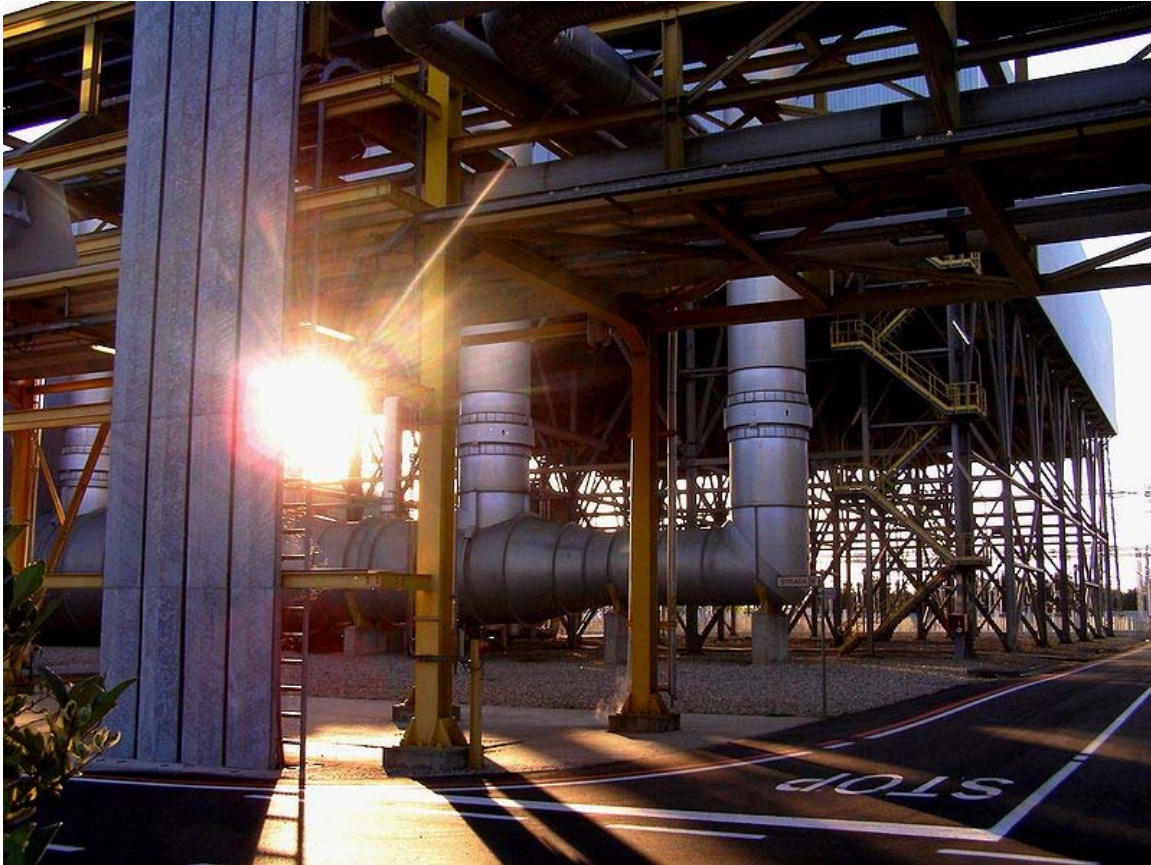
A cogeneration thermal power plant in Ferrera Erbognone (PV), Italy
