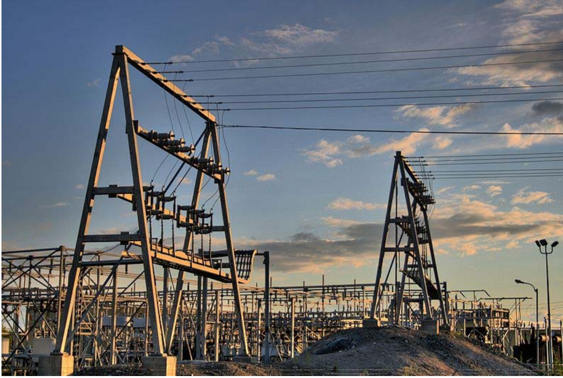
Substation near Yellowknife, in the Northwest Territories of Canada
