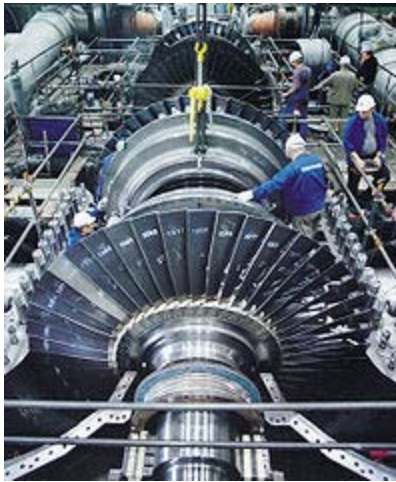
A steam turbine used to provide electric power.
