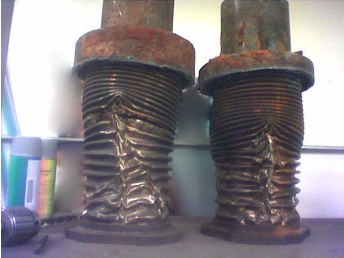
Expansion joints on a steam line that have been destroyed by steam hammer
