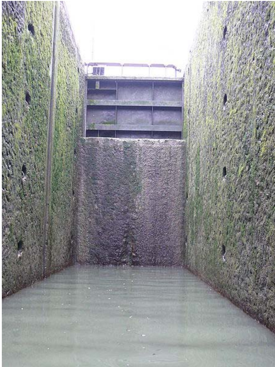
The cill exposed in the deep Pont de Flandre lock on the Canal Saint-Denis, Paris
