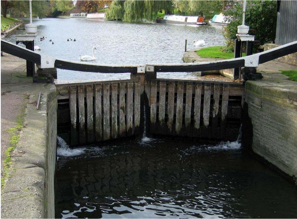
Top gate of a lock, showing the balance beams and paddle winding gear
