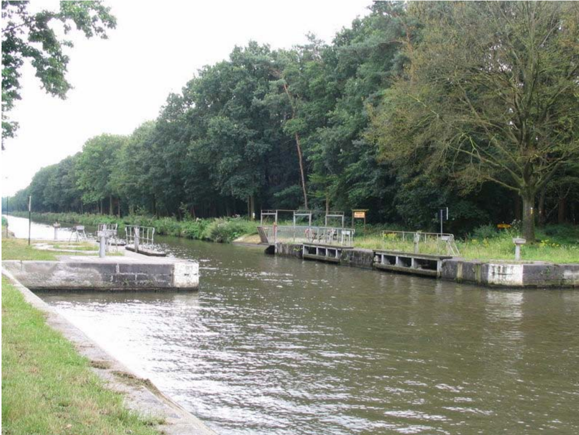
Bi-directional flood gates on the canal Schoten-Dessel, Belgium.
