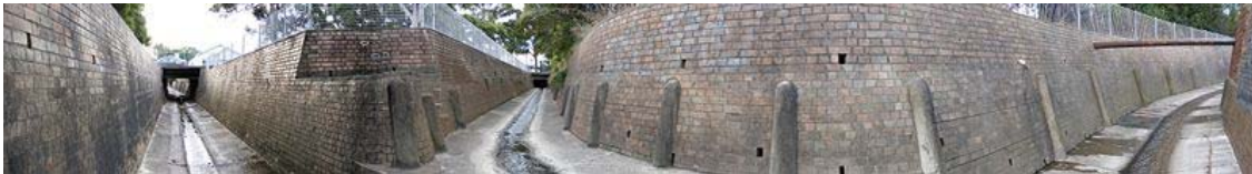
A typical drain in Bankstown, New South Wales.
