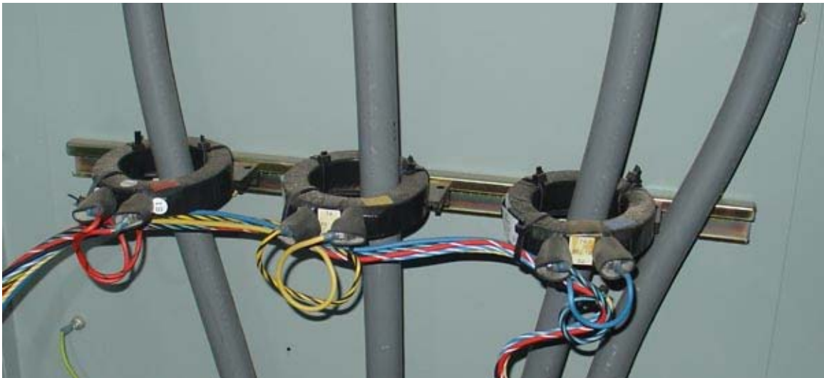
Current transformers used in metering equipment for three-phase 400 ampere electricity supply
