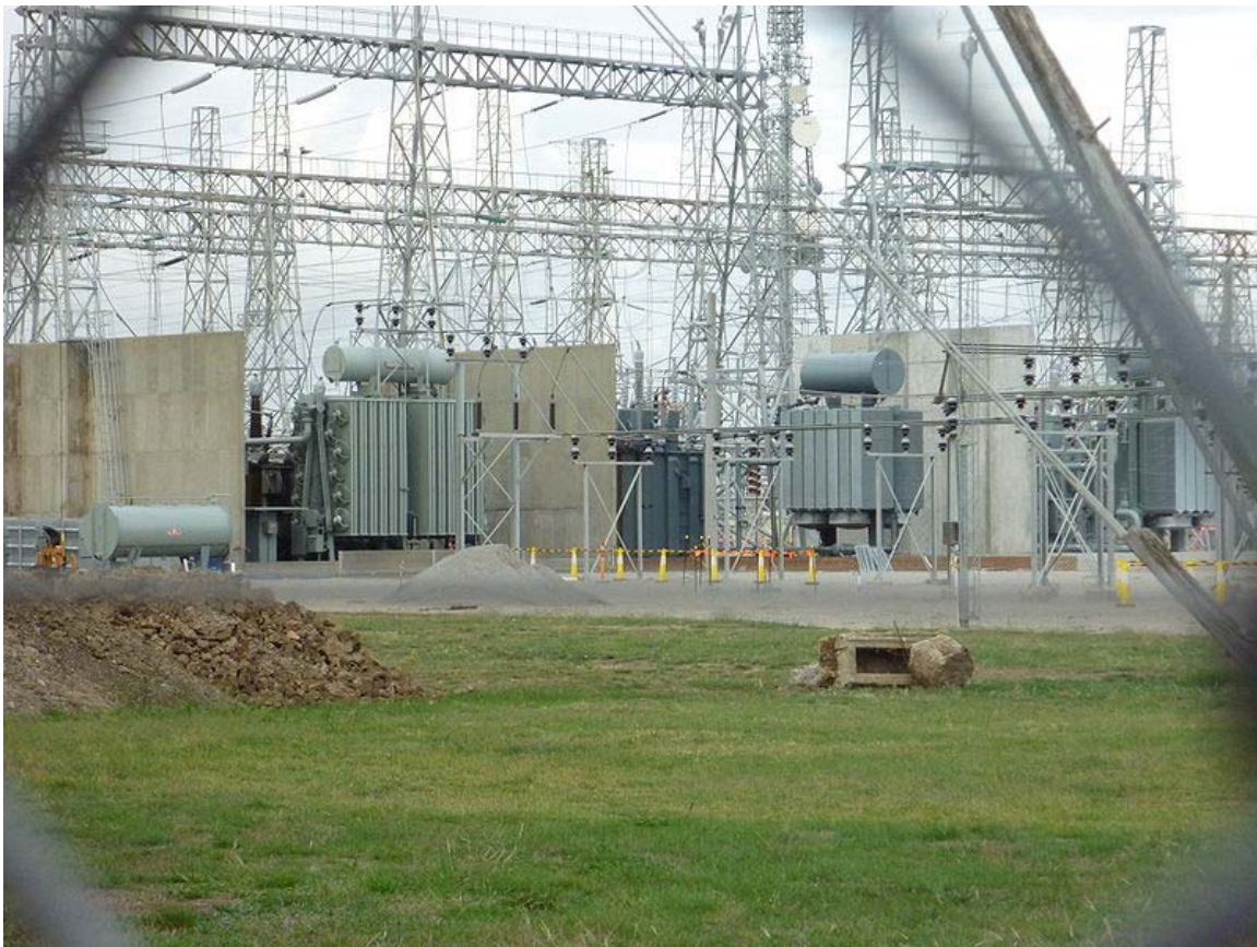
Image of an electrical substation in Melbourne, Australia showing 3 of 5 220kV/66kV transformers, each with a capacity of 185MVA
