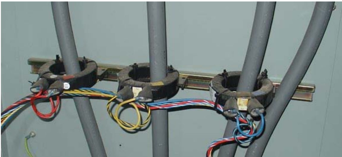
Current transformers used in metering equipment for three-phase 400 ampere electricity supply
