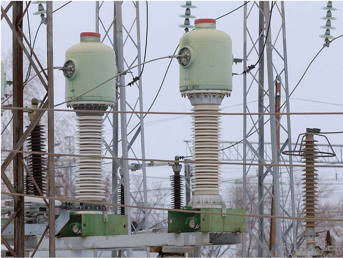
SF 6 110 kV current transformer TGFM series, Russia
