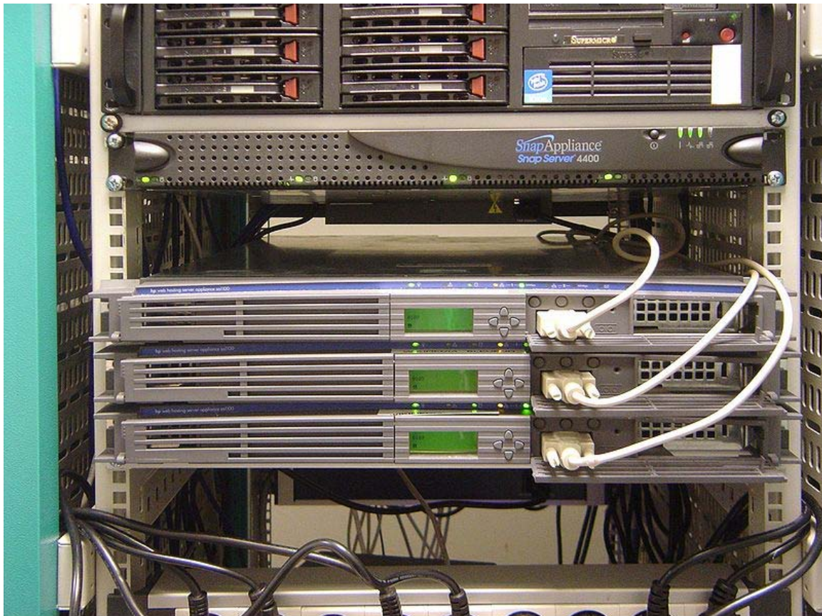
An example of "rack mounted" servers.
