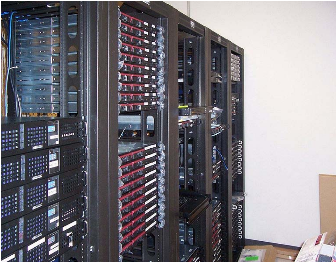
Multiple racks of servers, and how a data center commonly looks.
