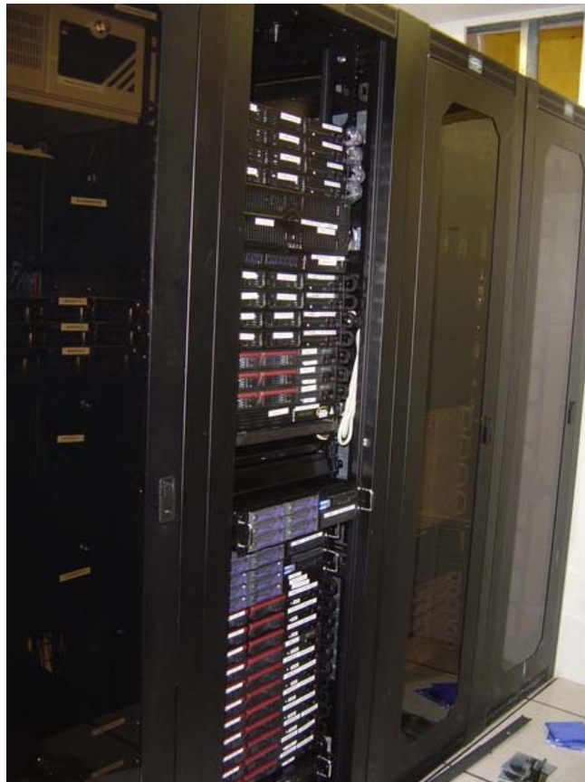
A row of racks in a server farm.
