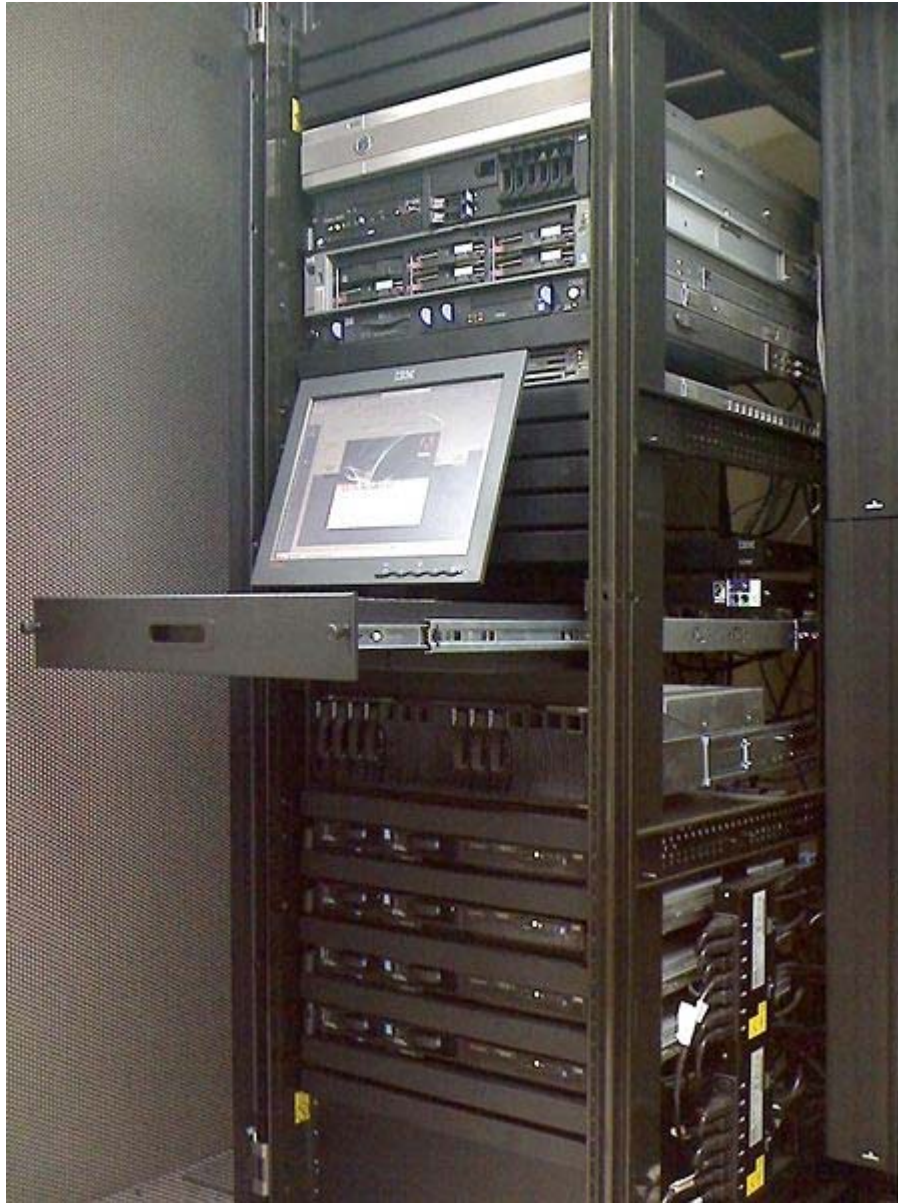
A typical server rack, commonly seen in colocation.
