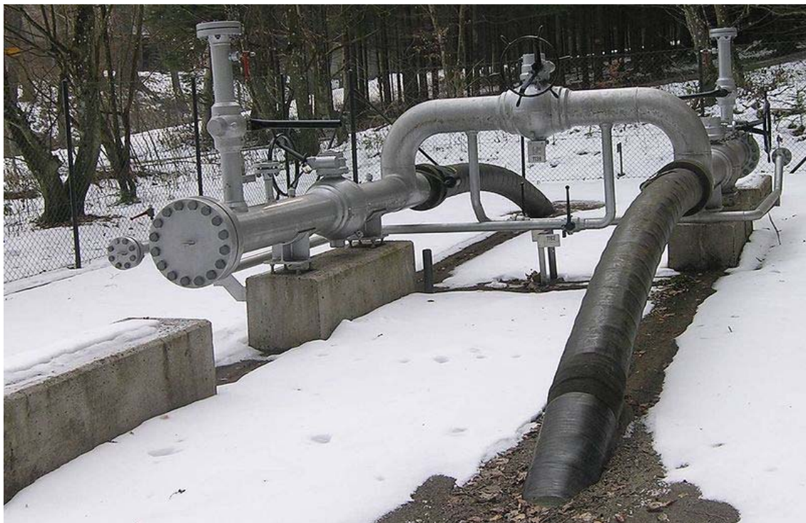
A "Pig" launcher/receiver, belonging to the natural gas pipeline in Switzerland.
