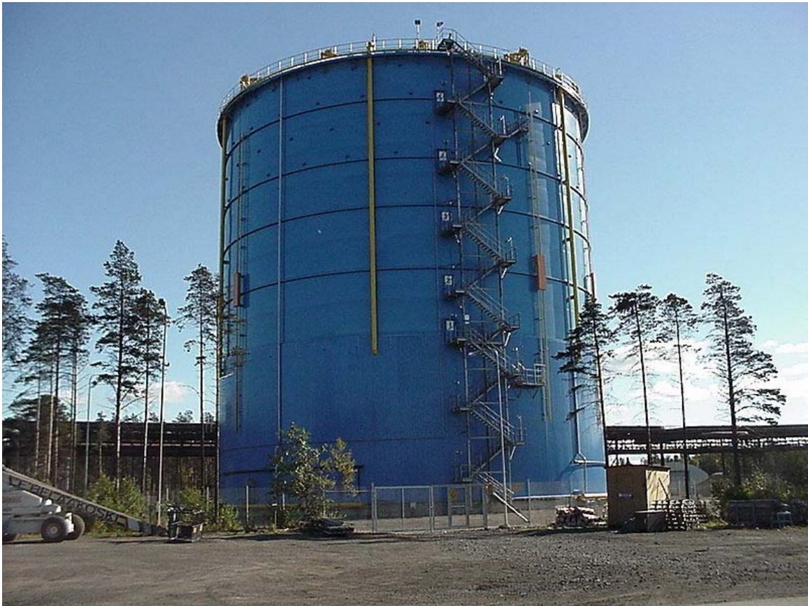
30,000m 3 BF Gas holder at Rautaruukki Steel in Finland.
