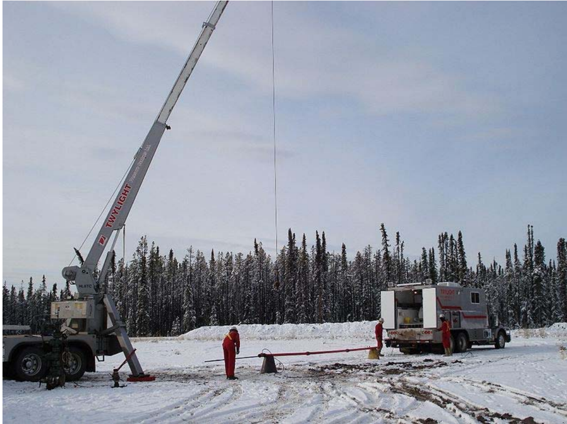
Wireline Truck with drum (inside)
