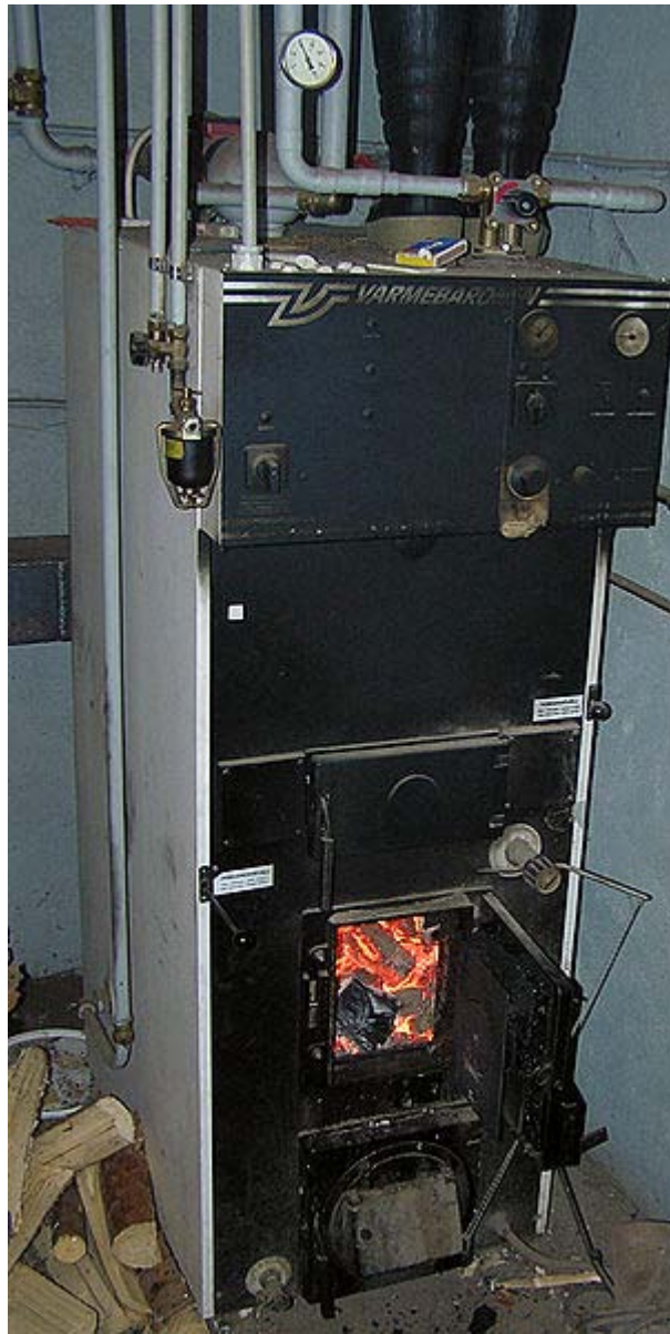
Central heating unit
