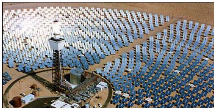
The Solar Two solar-thermal power project. Every mirror in the field of heliostats reflects sunlight continuously onto the receiver on the tower.
