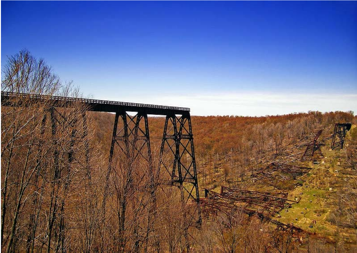
The Kinzua Bridge after it collapsed
