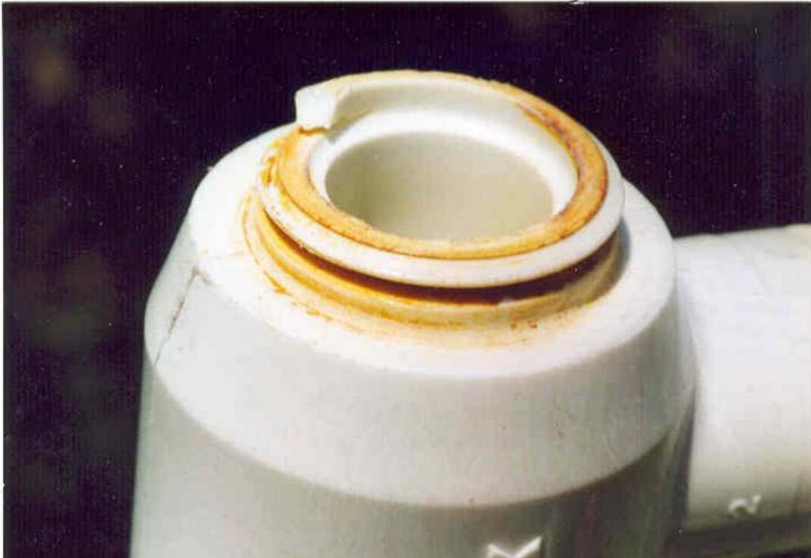
chlorine attack of acetal resin plumbing joint
