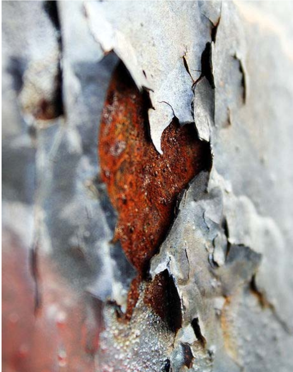
Flaking paint, exposing a patch of surface rust on sheet-metal
