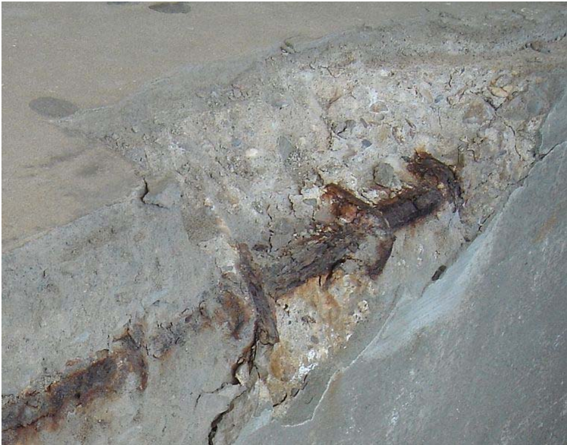
Carbonation-initiated deterioration of concrete at Hippodrome Wellington, Belgium.
