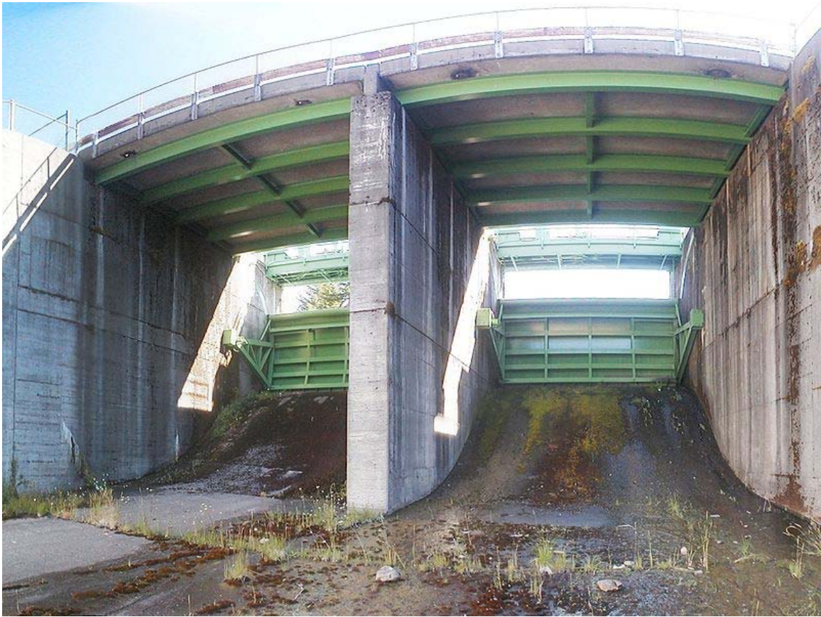
Tainter gates and spillway
