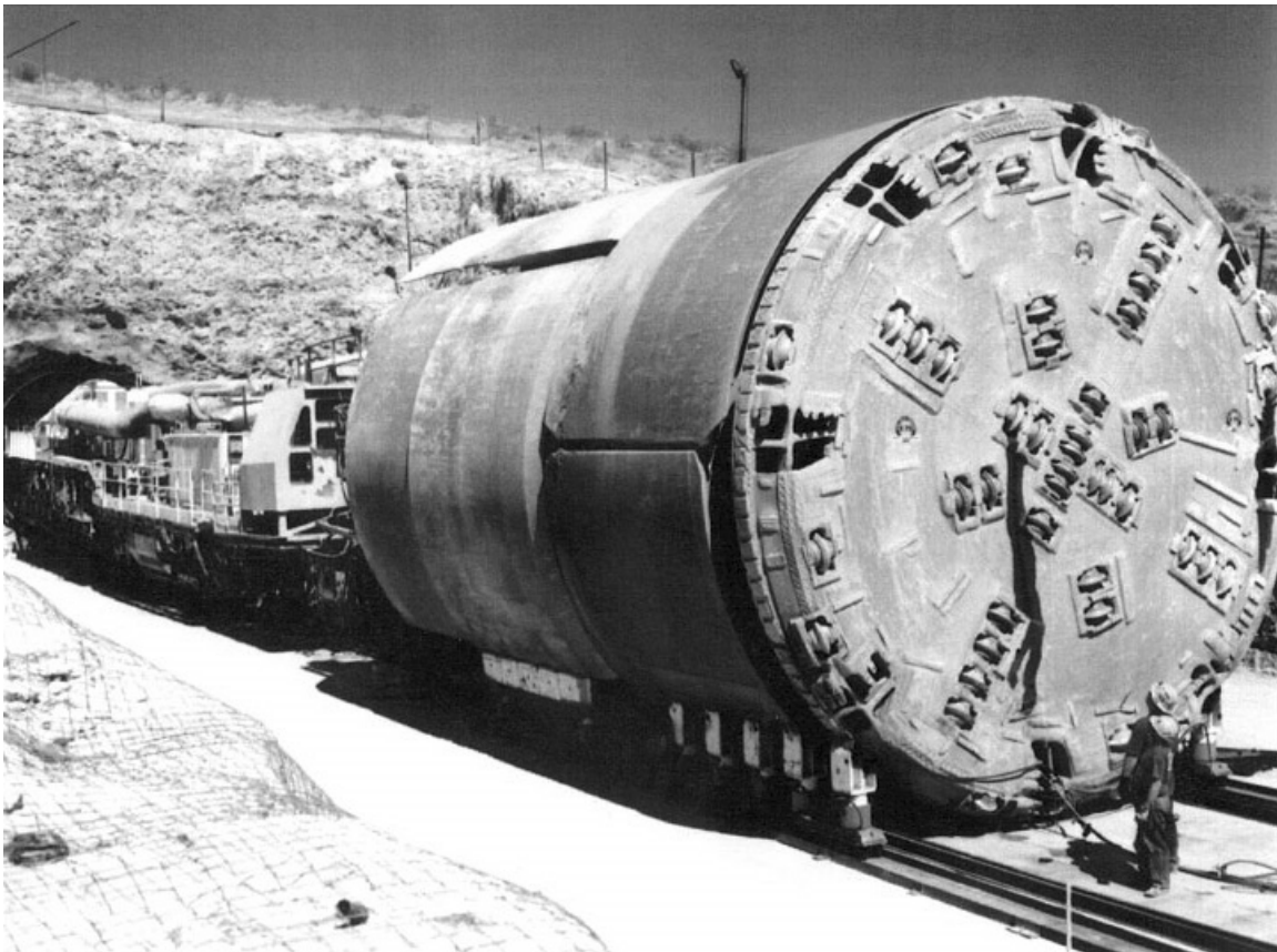
A tunnel boring machine that was used at Yucca Mountain nuclear waste repository
