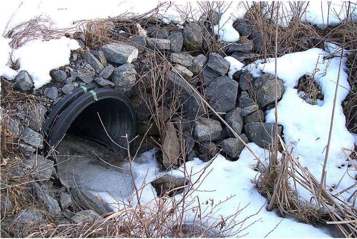
Polymer drainage culvert
