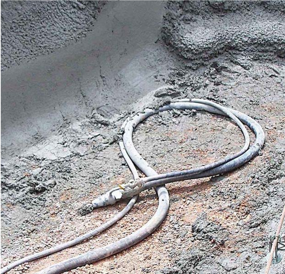
Shotcrete nozzle with 75 mm concrete hose from line pump and 20 mm compressed air line.
