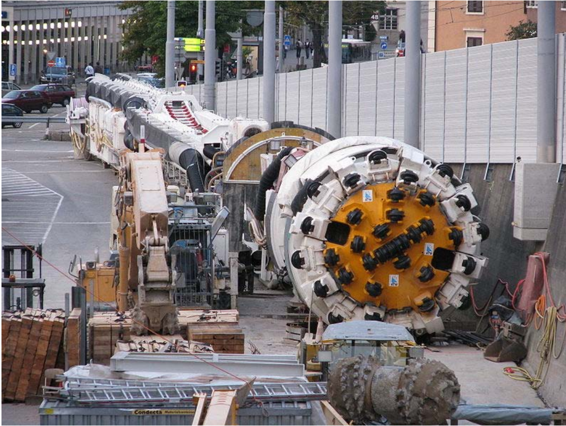
Tunnel boring machine at the site of Weinberg tunnel Altstetten-Zürich-Oerlikon near Zürich Oerlikon train station.
