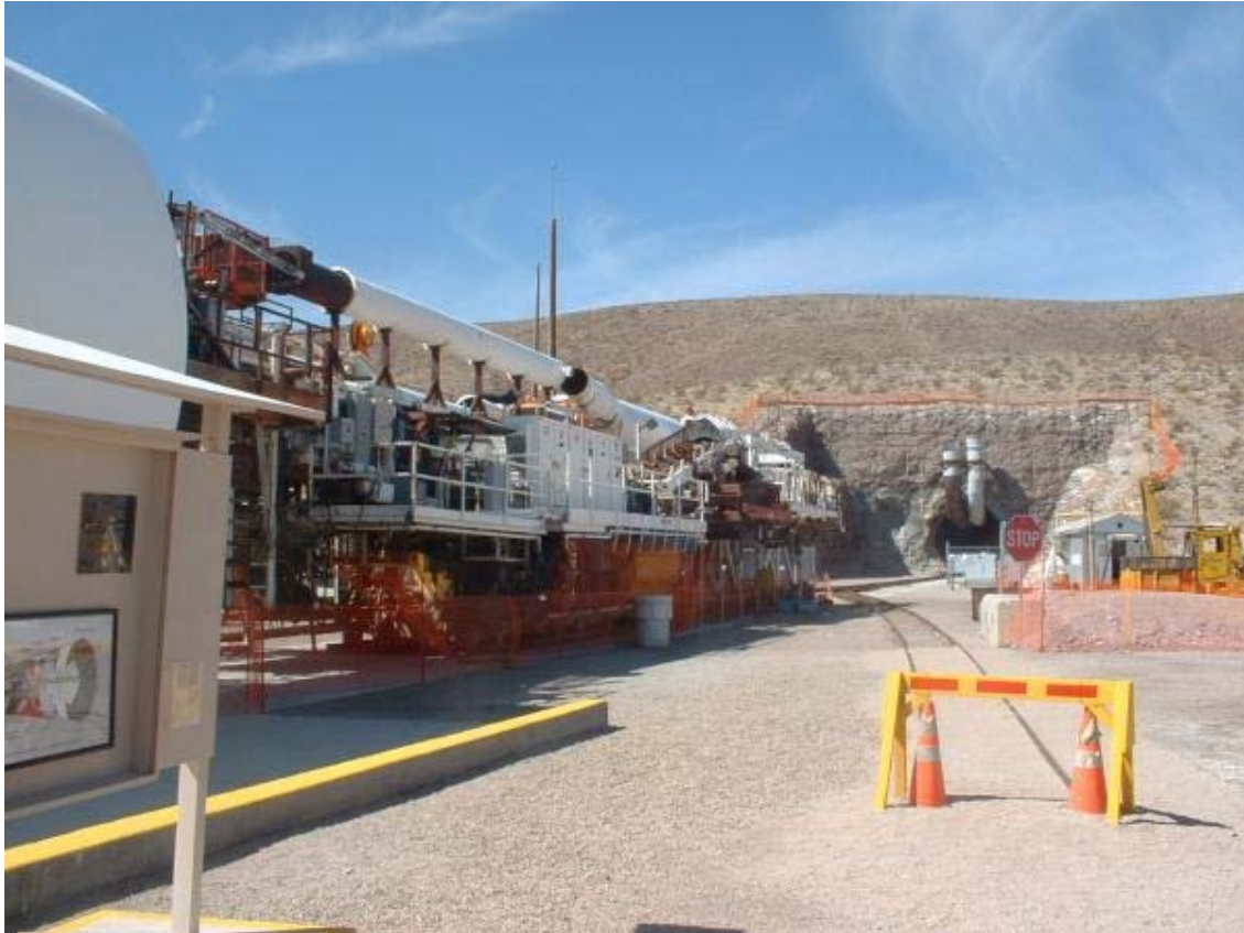
The support structures at the rear of a TBM. This machine was used to excavate the main tunnel of the Yucca Mountain nuclear waste repository in Nevada.
