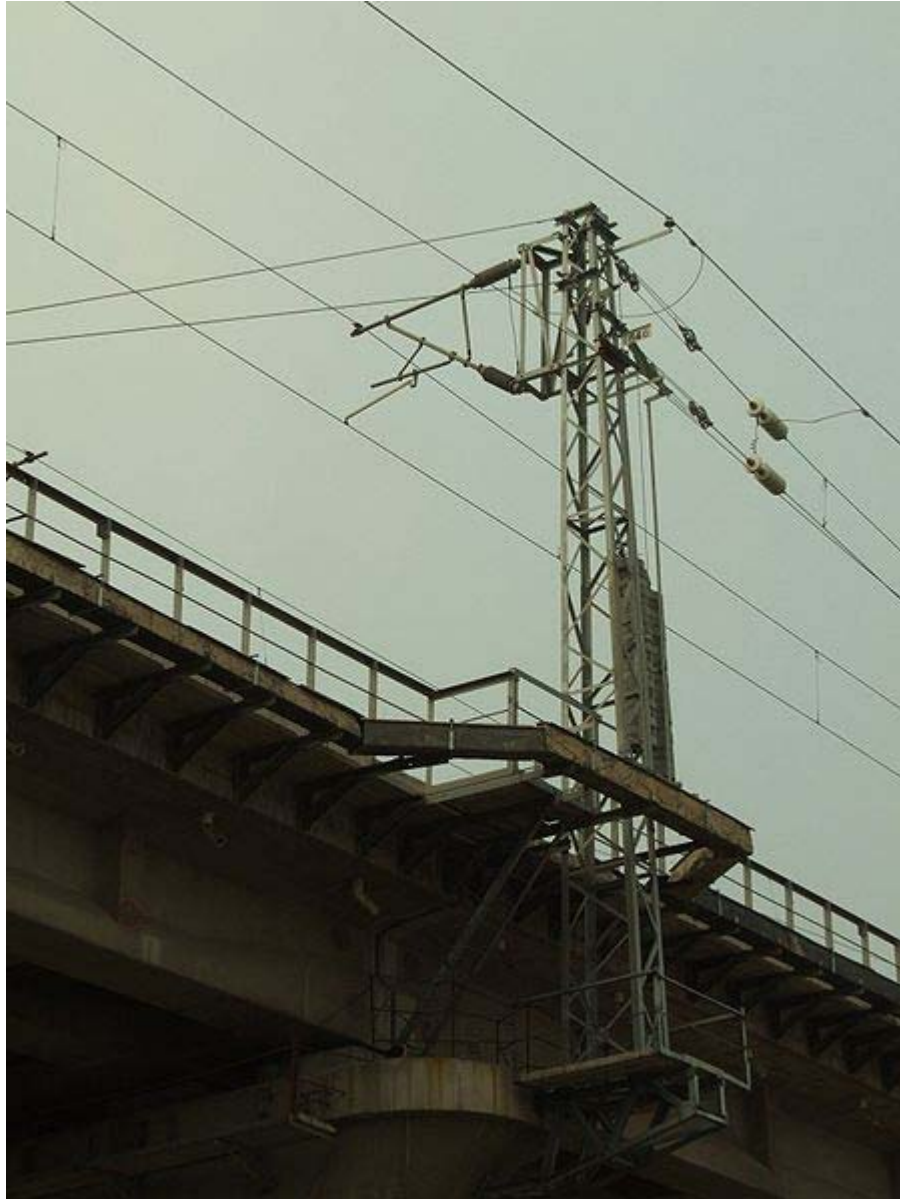
The overhead lines in China
