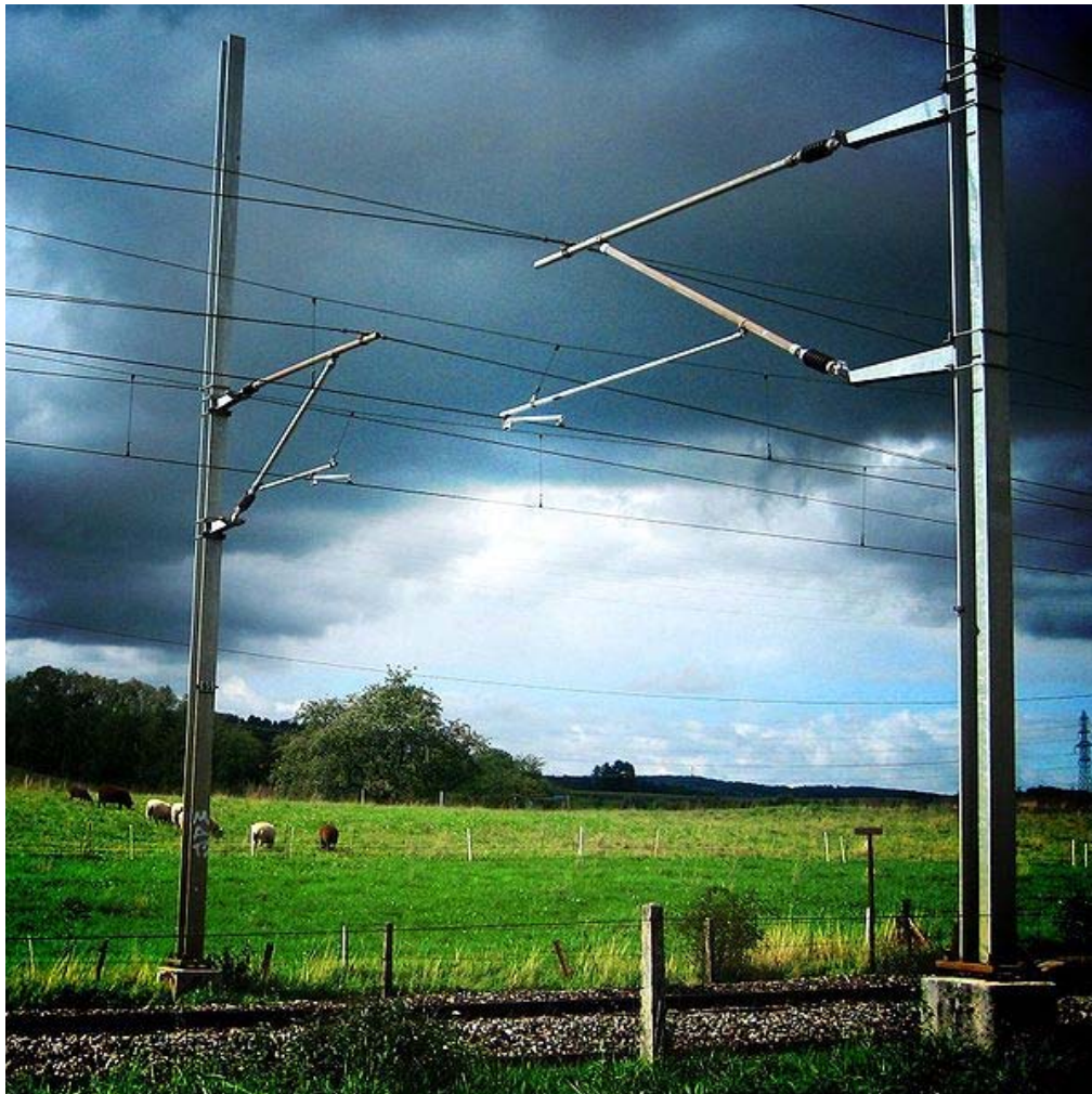
Overhead lines on Swiss Federal Railways
