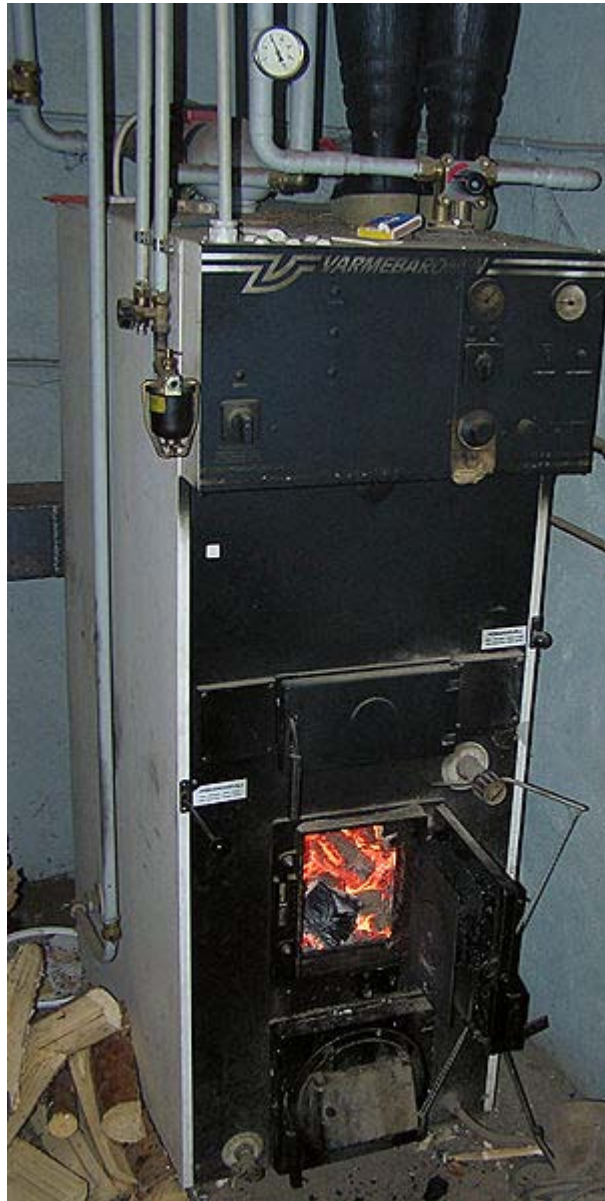
Central heating unit
