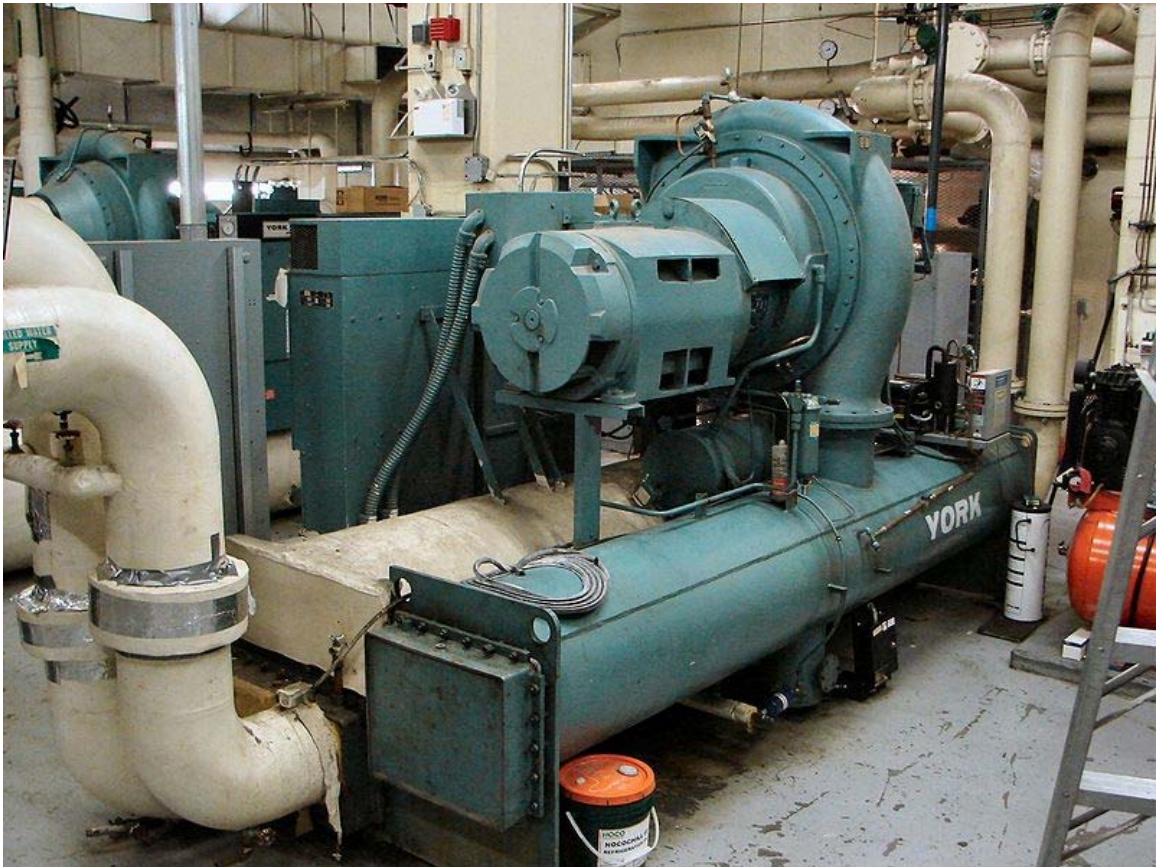
York International water-cooled chiller.
