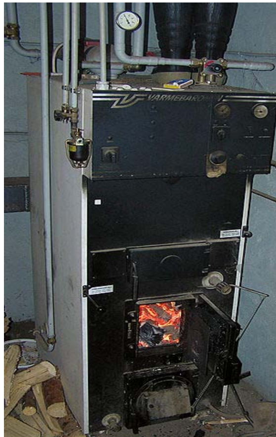
Central heating unit
