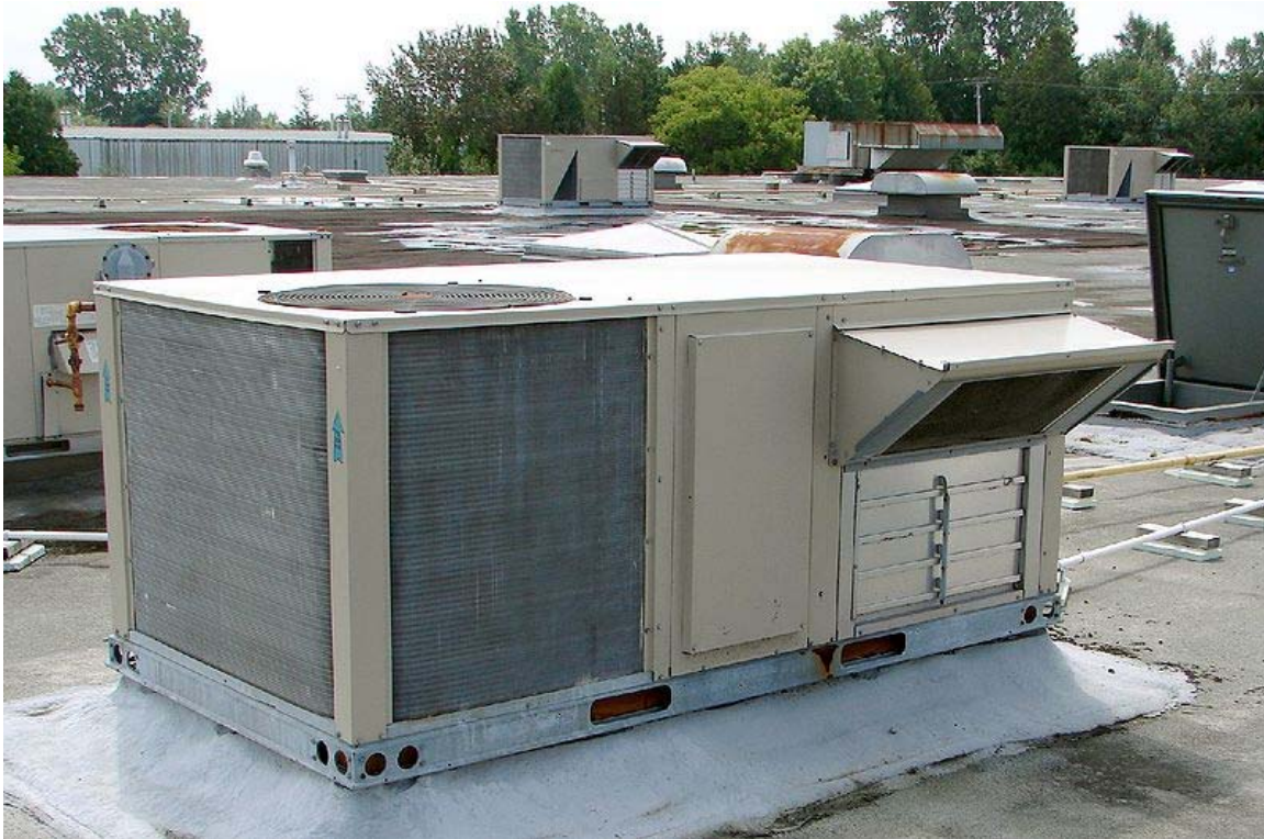
A rooftop packaged unit or RTU
