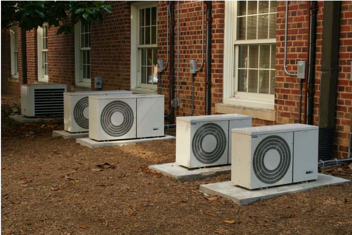
Air conditioning units outside a classroom building at the University of North Carolina in Chapel Hill, North Carolina
