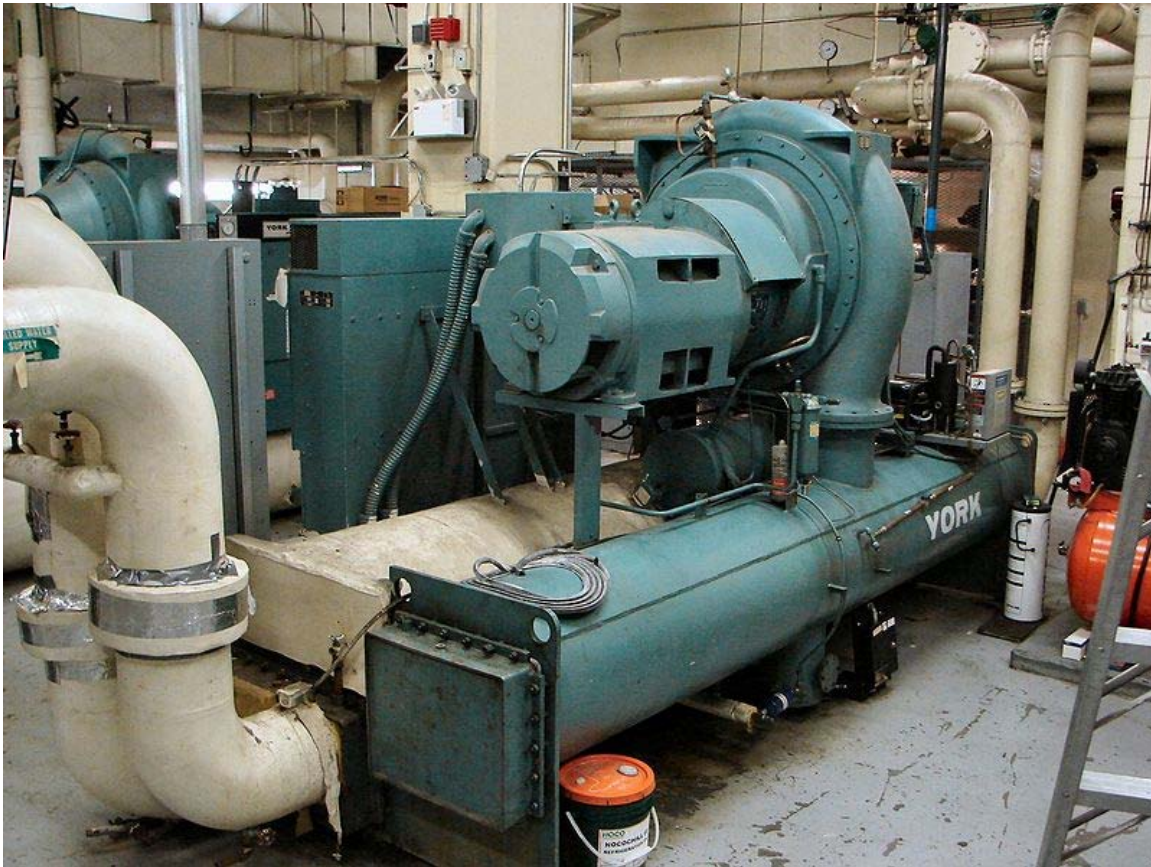
Figure 5: Commercial water cooled liquid chiller installation for building air conditioning
