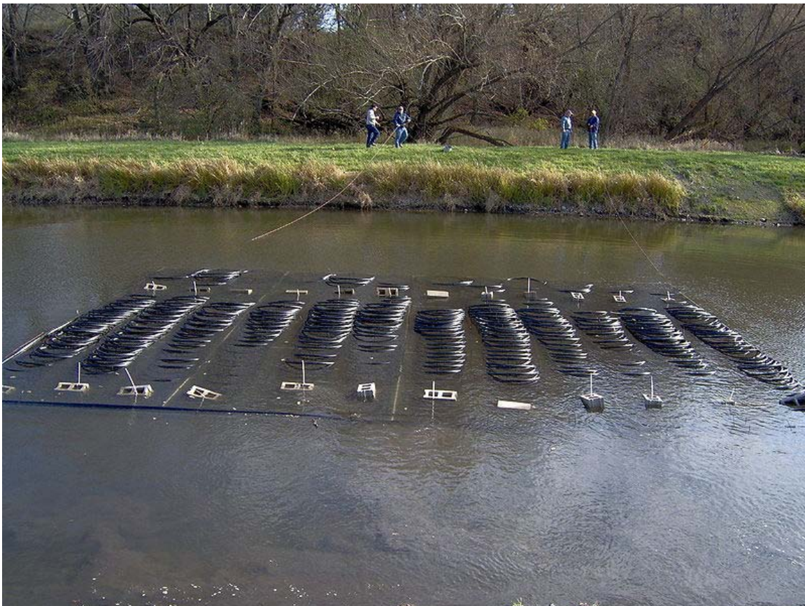
12-ton pond loop system being sunk to the bottom of a pond
