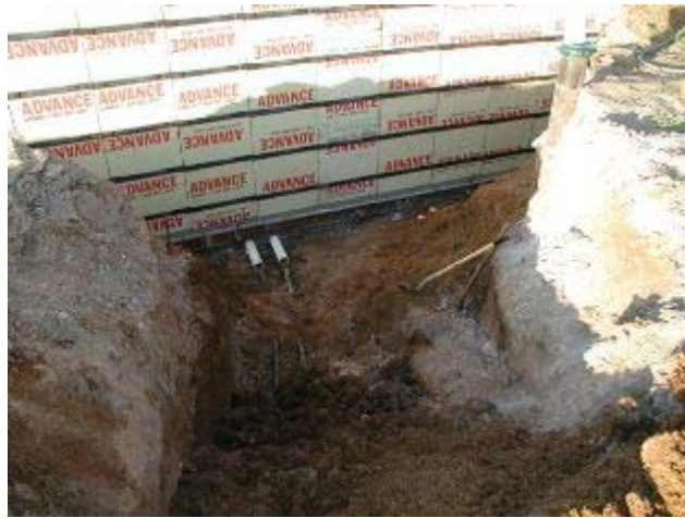
Ground source heating and cooling
