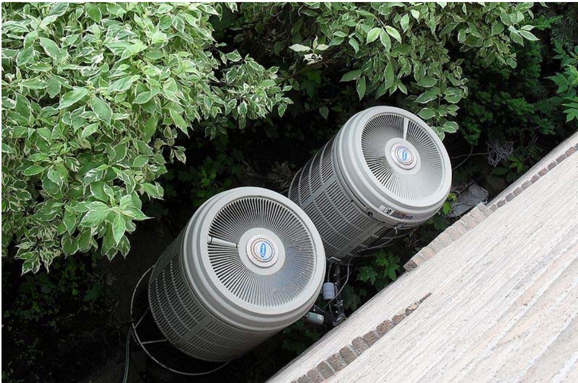
Outdoor components of a residential air-source heat pump
