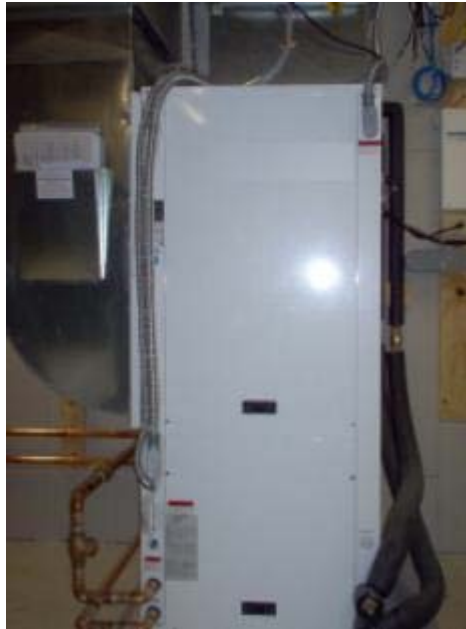
Liquid-to-air heat pump
