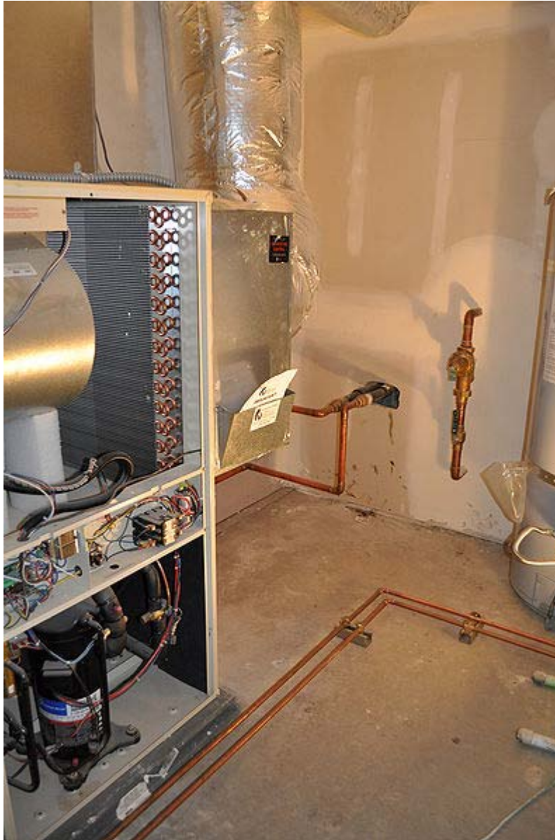
Ground source heating and cooling
