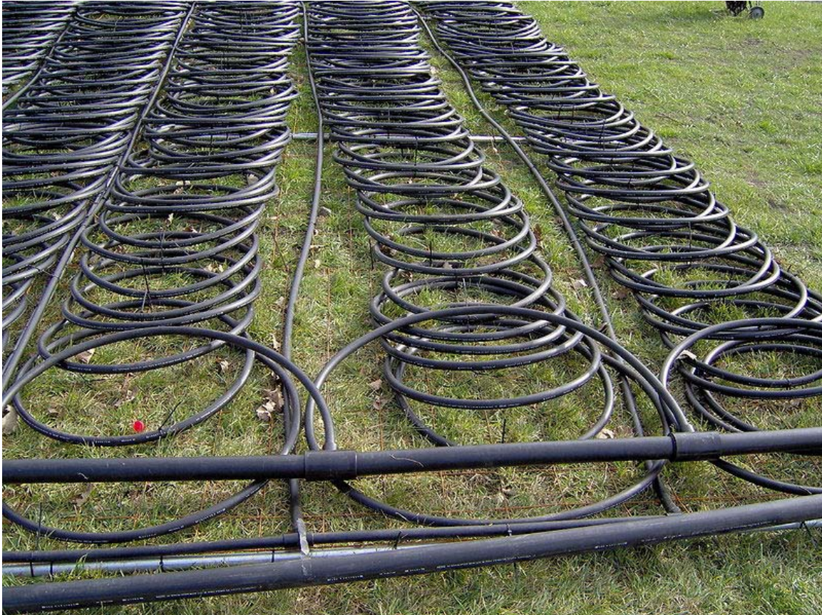
Loop field for a 12-ton system (unusually large for most residential applications)
