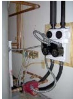
An installed liquid pump pack
