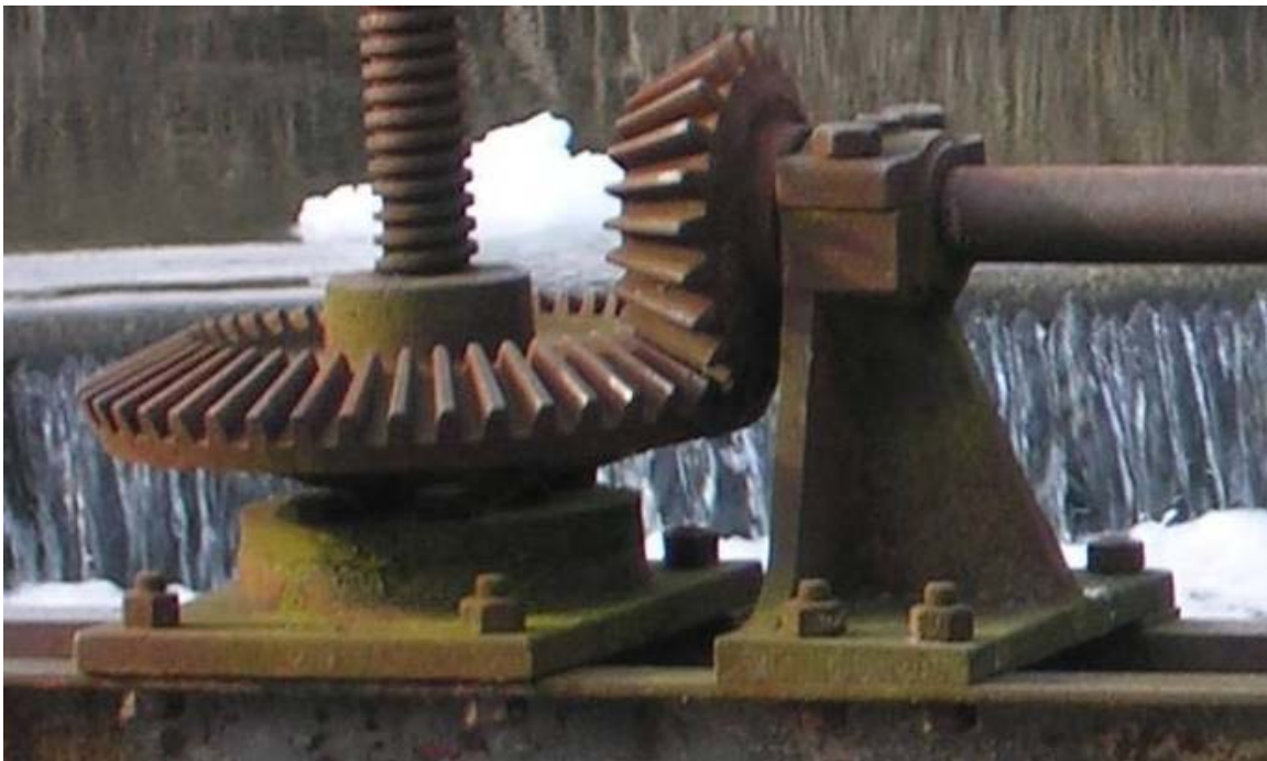
Bevel gear lifts floodgate by means of central screw.
