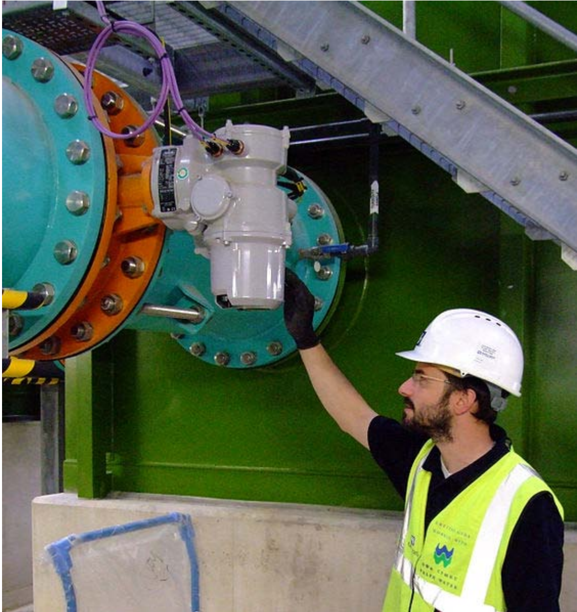
Electric part-turn actuator on a butterfly valve
