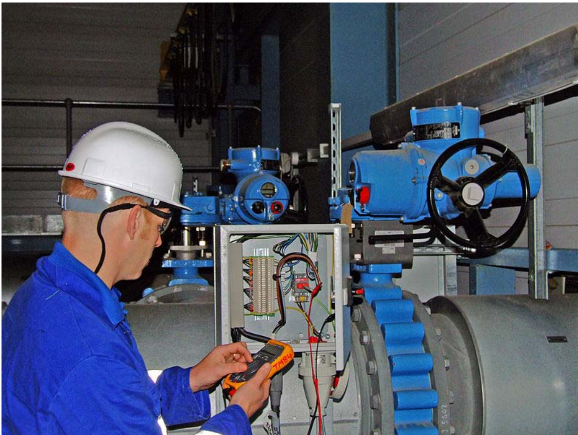
Electric actuator on a valve in a power plant
