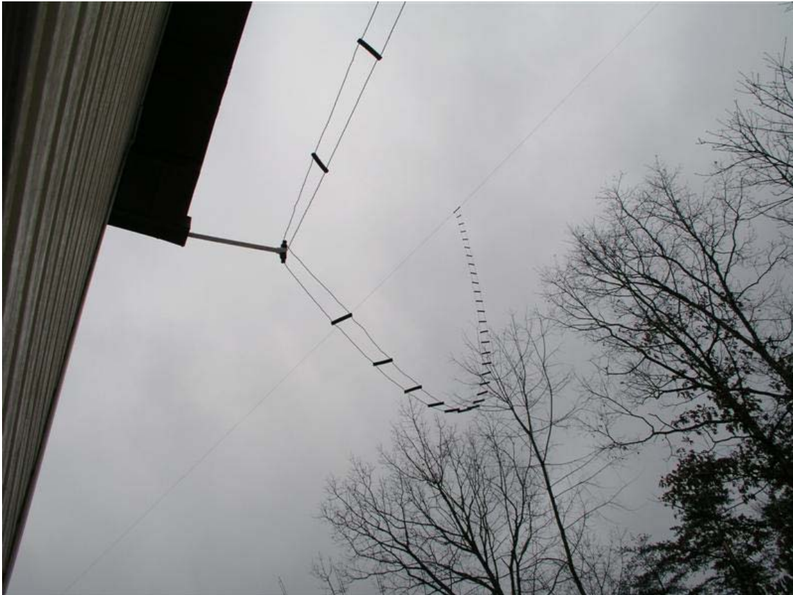
600 Ohm "Ladder line" on the outside of a building.
