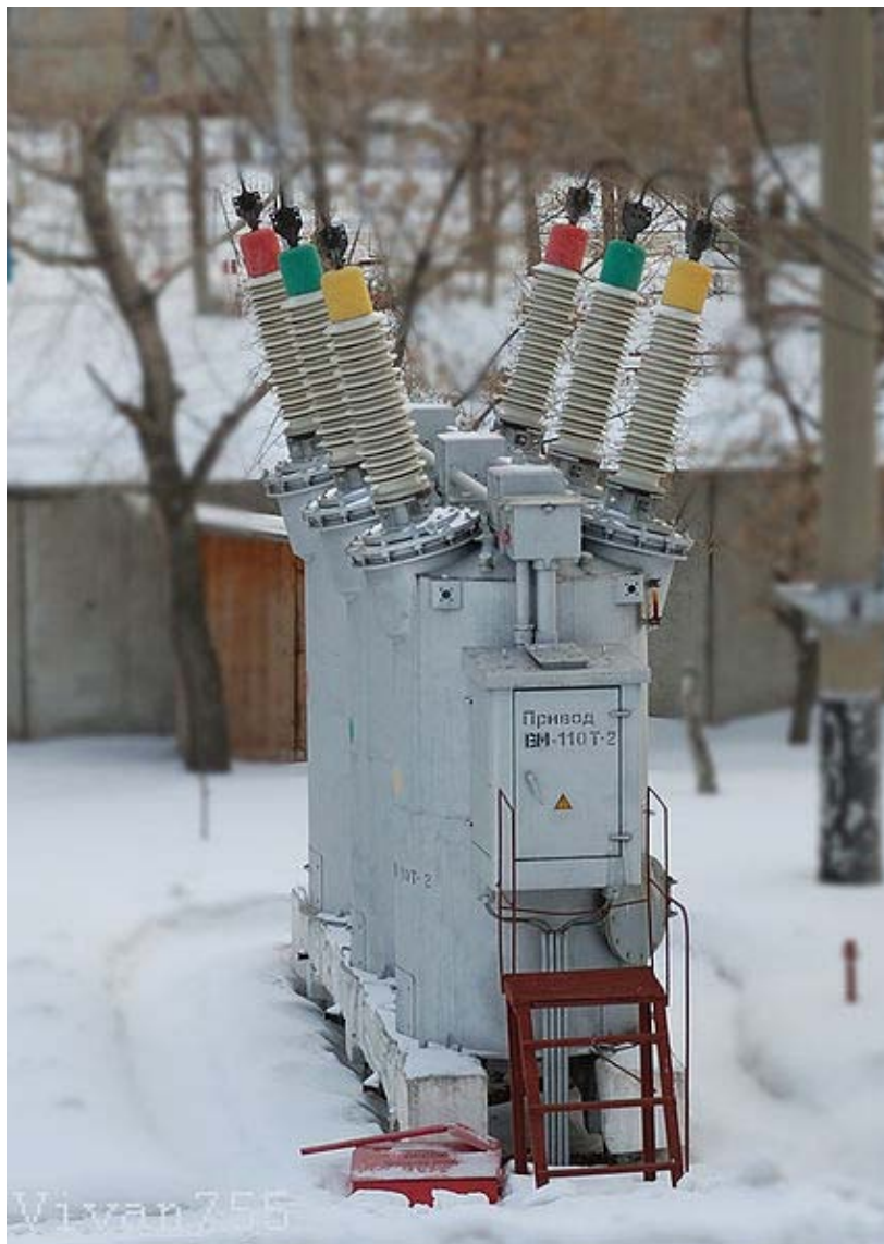
Russian 110 kV oil circuit breaker
