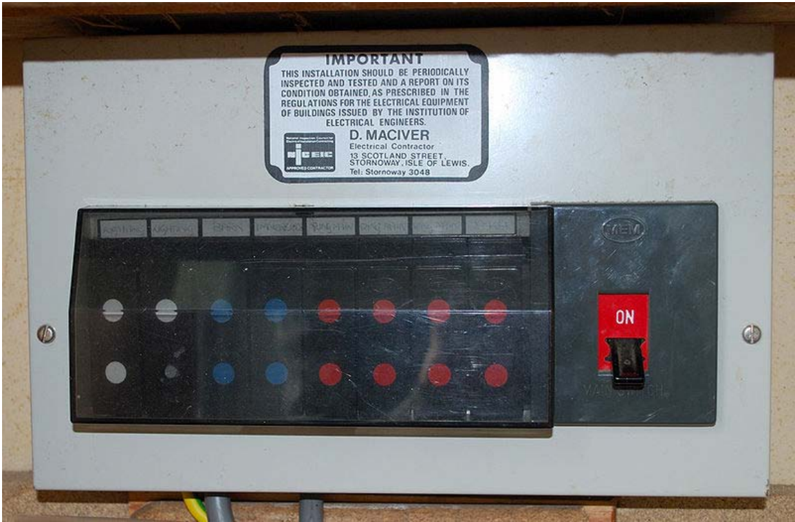
1970s MEM rewirable fuse box (covered)
