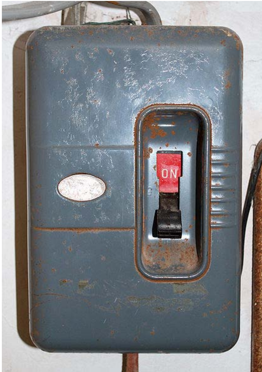
1950s MEM rewirable fuse box (covered)
