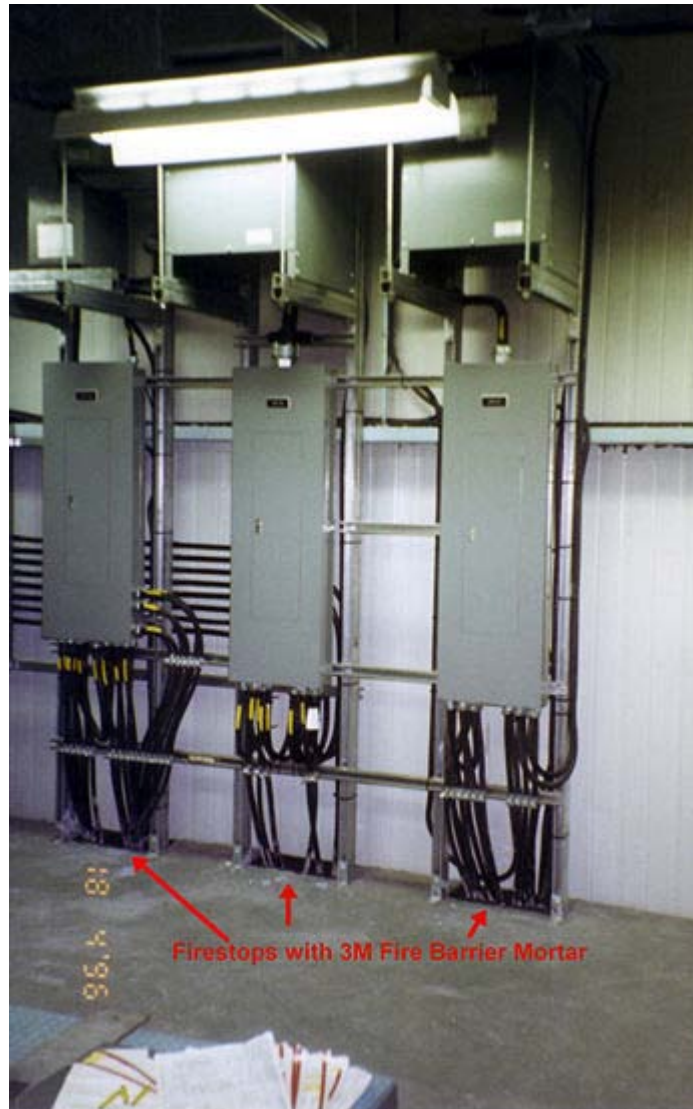
Electrical panels in an electrical service room at St. Mary's Pulp and Paper, Sault Ste. Marie, Ontario, Canada, April 1996
