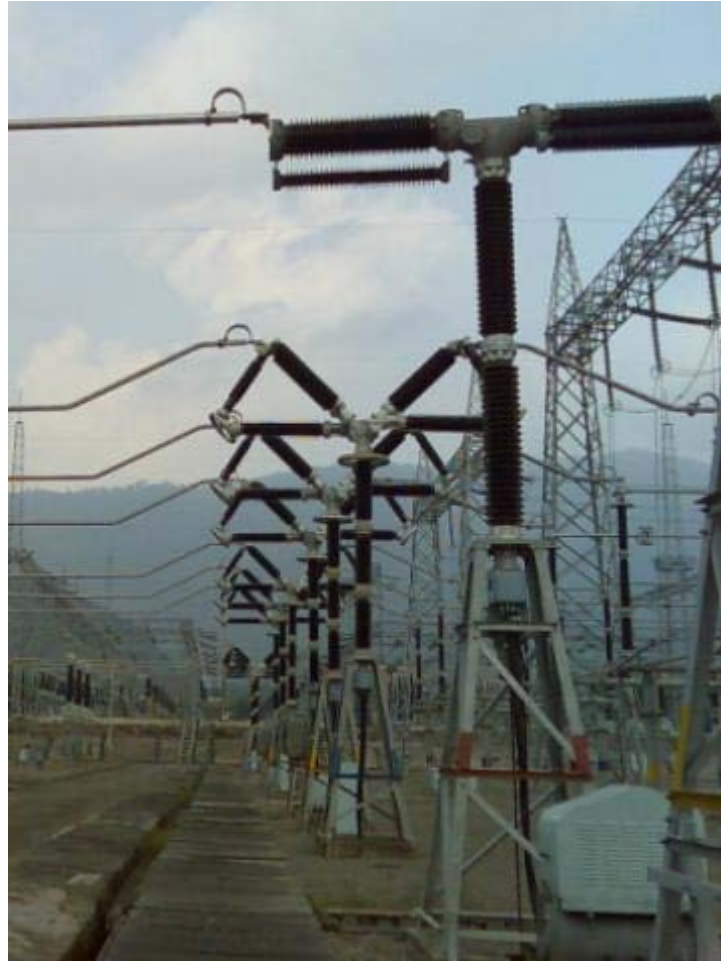
400 kV SF 6 live tank circuit breakers
