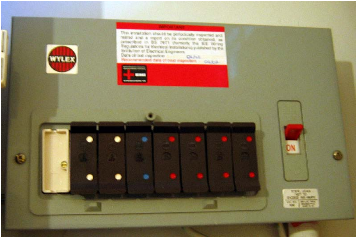
Wylex fuse box
