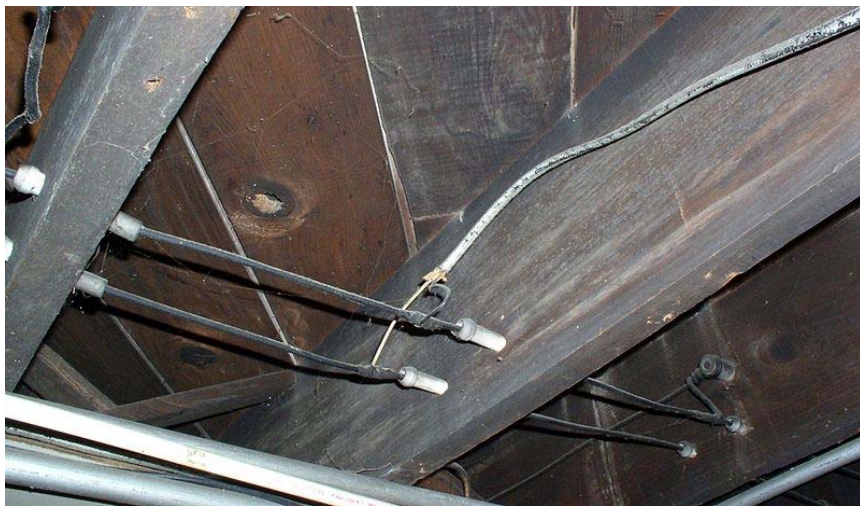
Wiring running through tubes, and turning a corner supported by a knob. Notice the direct splice with more modern (1950s-era) NonMetallic sheathed cable. This type of connection is forbidden by NEC electrical code, and other methods should have been used.
