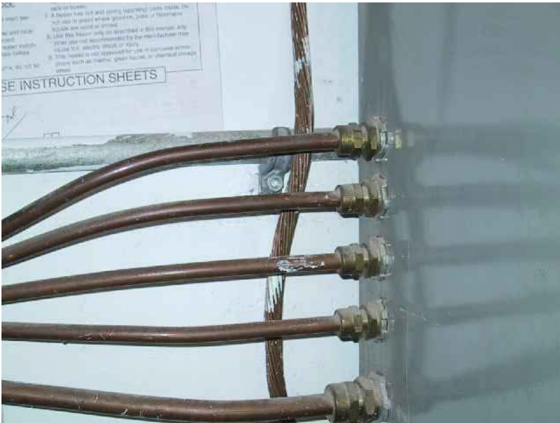
Mineral insulated cables at a panel board
