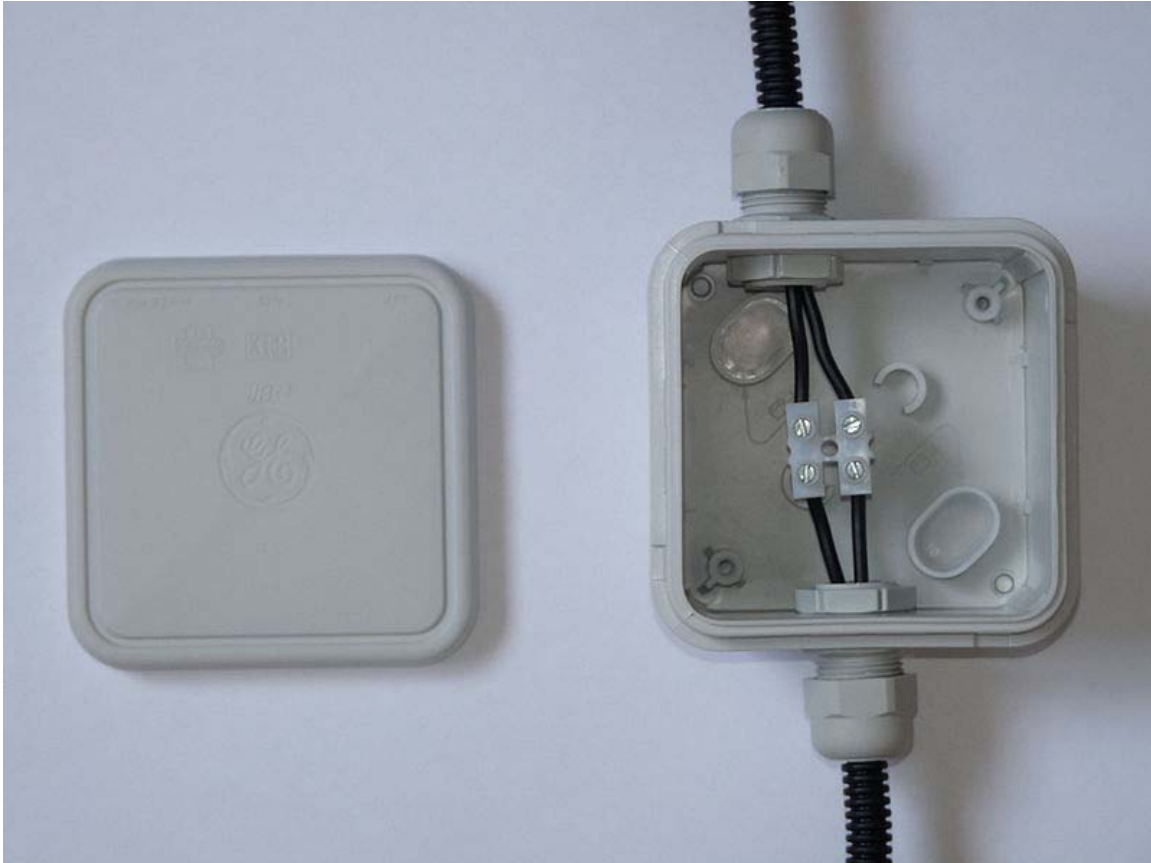
Wiring in extremely-wet conditions
