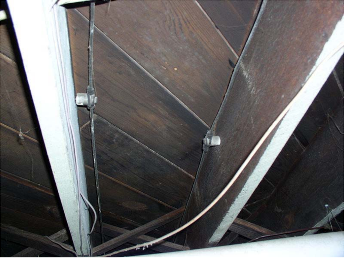
Knobs supporting long runs of wire
