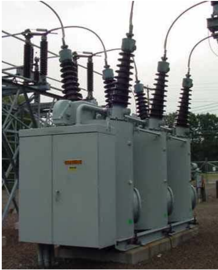
115 kV bulk oil circuit breaker
