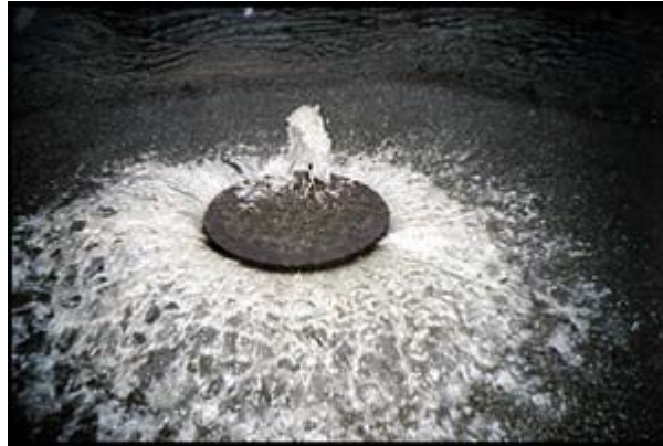
A manhole cover unable to contain a sanitary sewer overflow
