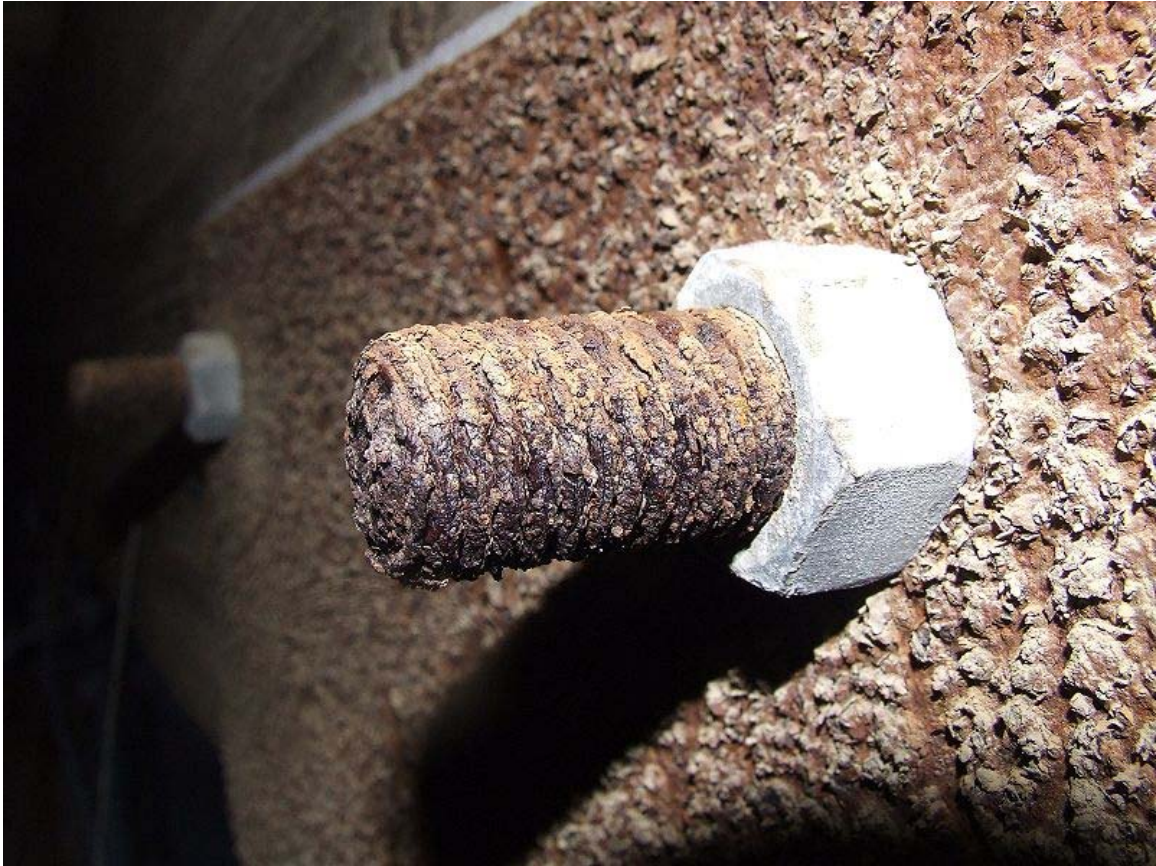
Corrosion on exposed metal.
