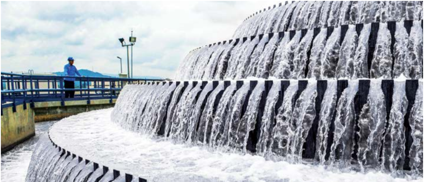
Aerator in Semangar Water Treatment Plant
