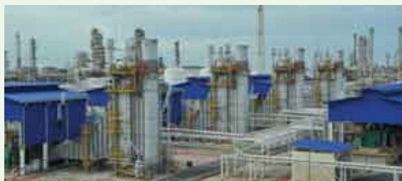
A cogeneration unit located at PP(M)SB
